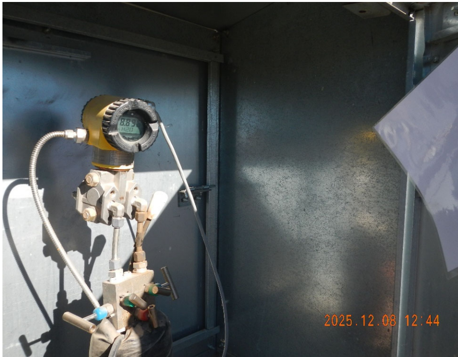
3. Gas Meter inside Flowline mounted Meter Box.
