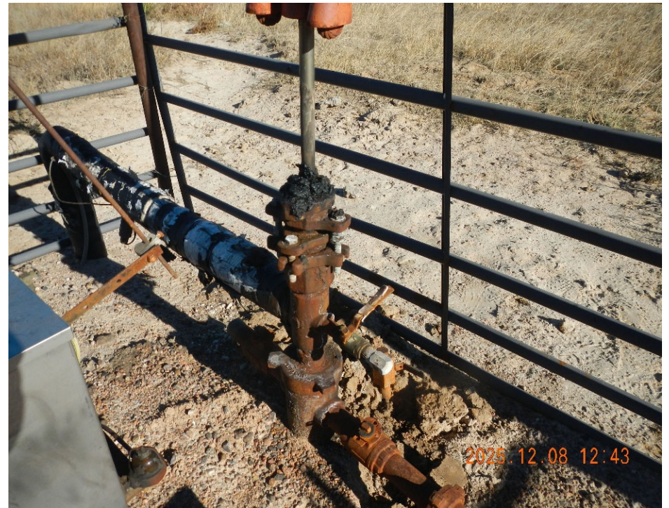
2. View of wellhead.
