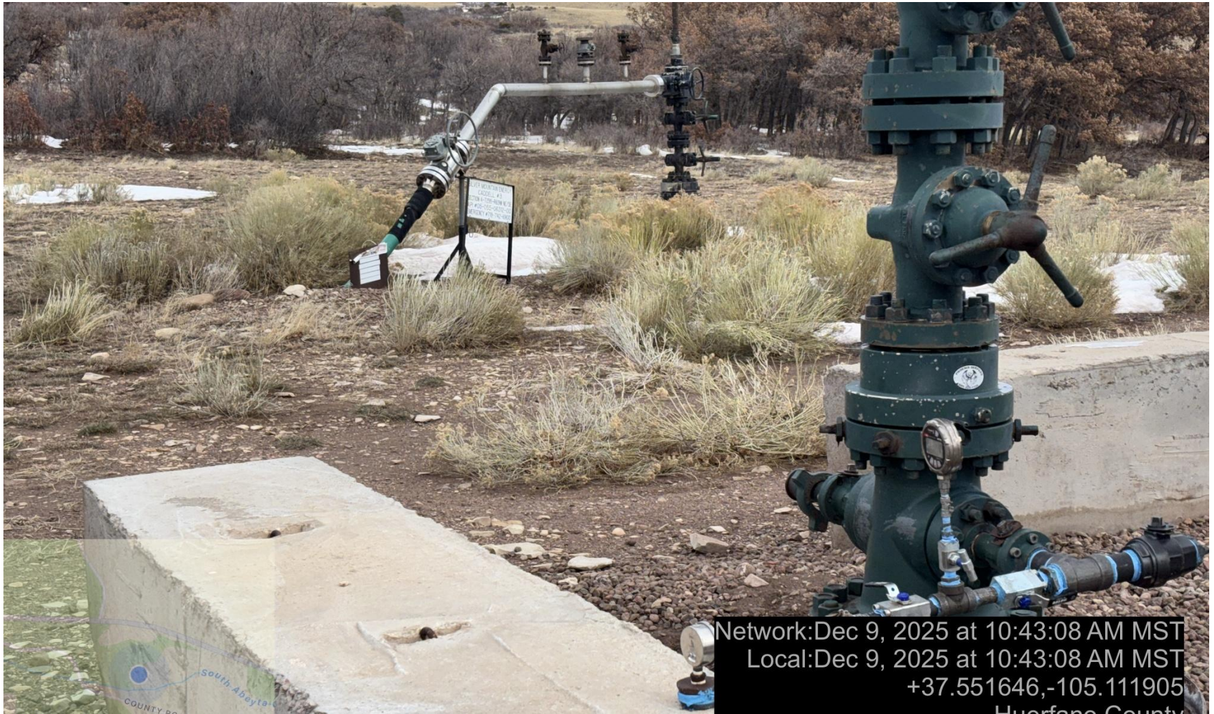
PHOTO 3: WELLHEAD AND EQUIPMENT.
