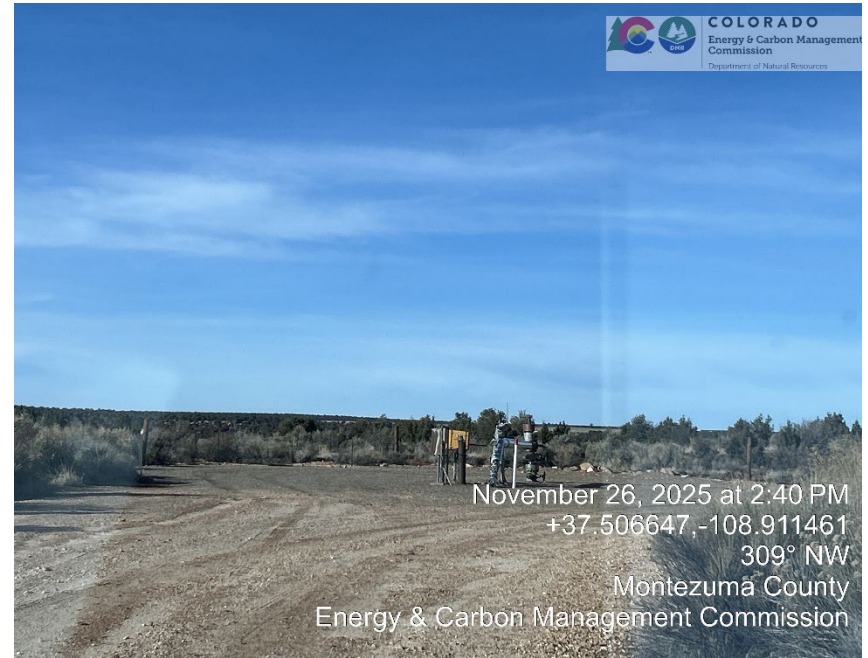
2. Well head and meter. Down fence is on left.
