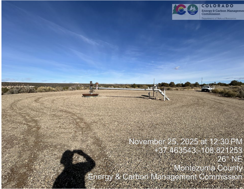
3. View of well and meter run.
