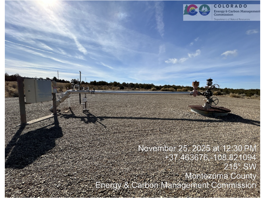
4. View of well and meter run.
