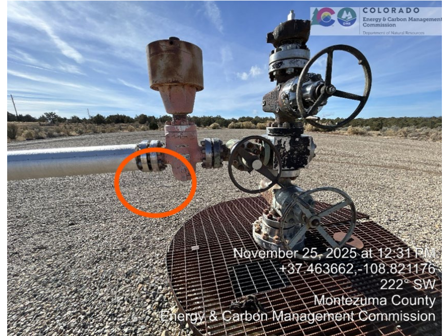
6. View of well head. Note disconnected wires.
