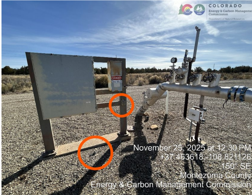
5. View of meter and control box. Note that wires and conduit have been clipped at ground level and at meter box.
