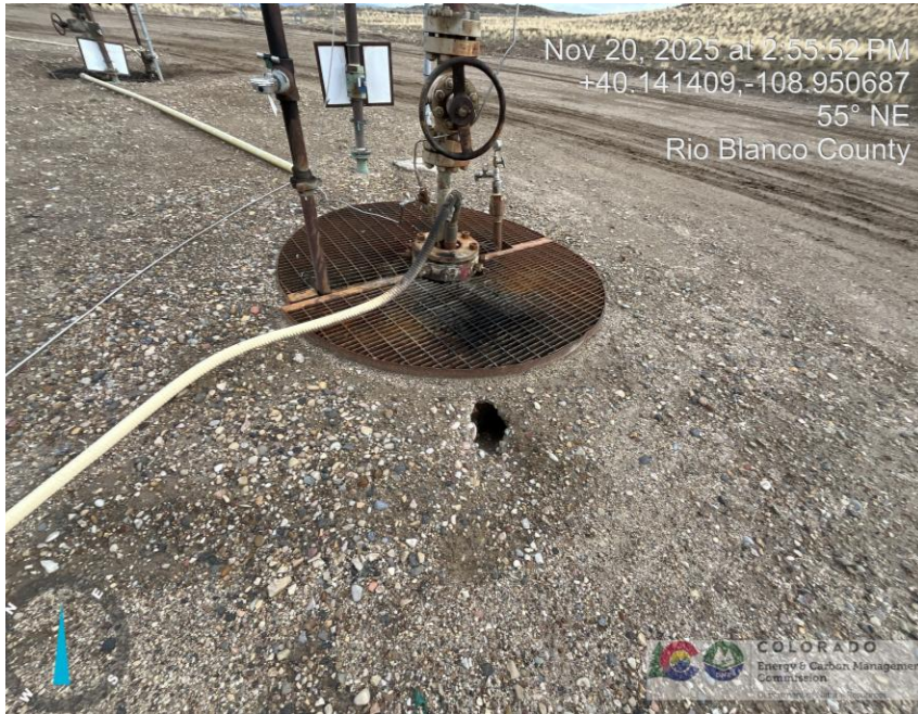
Photo # 4441 Tunnel erosion near D.F. ROOTH #5 wellhead/needs maintenance.
