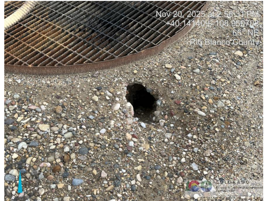
Photo # 4443 Tunnel erosion near D.F. ROOTH #5 wellhead/needs maintenance.
