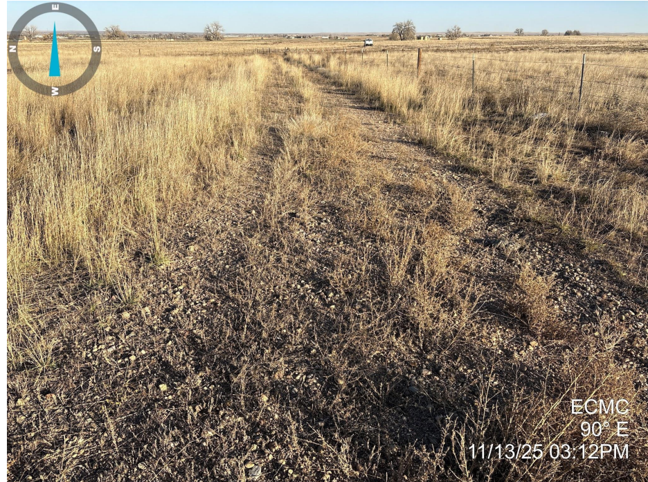
Photo 4. Photo taken of the access road to the well location, facing east, away from the location. Photo illustrates that final reclamation activities have not taken place along the access road and gravel remains.
