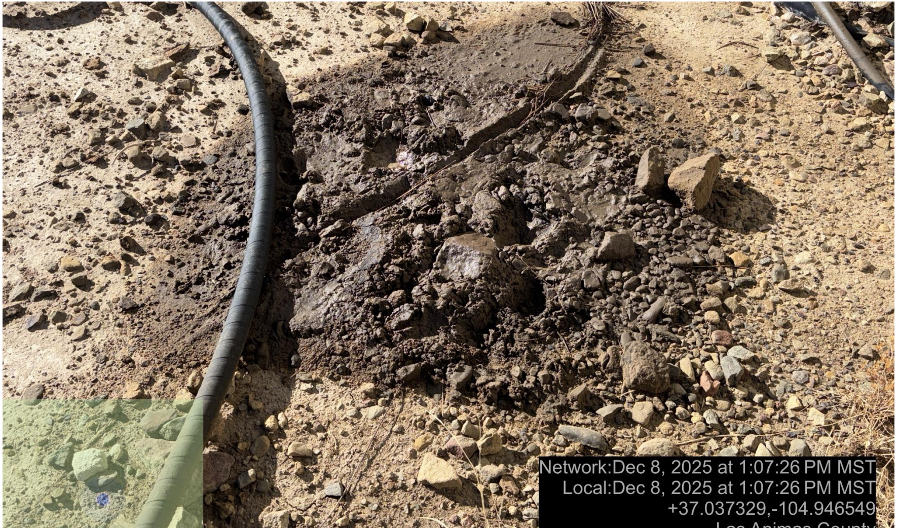
PHOTO 4: IMPACTED SOIL BETWEEN PRIME MOVER AND WELLHEAD. Conduct maintenance on equipment, cleanup stained material and review self inspection processes. COMPLY WITH RULE 1002,(2).D. CA DATE 12-15-2025.
