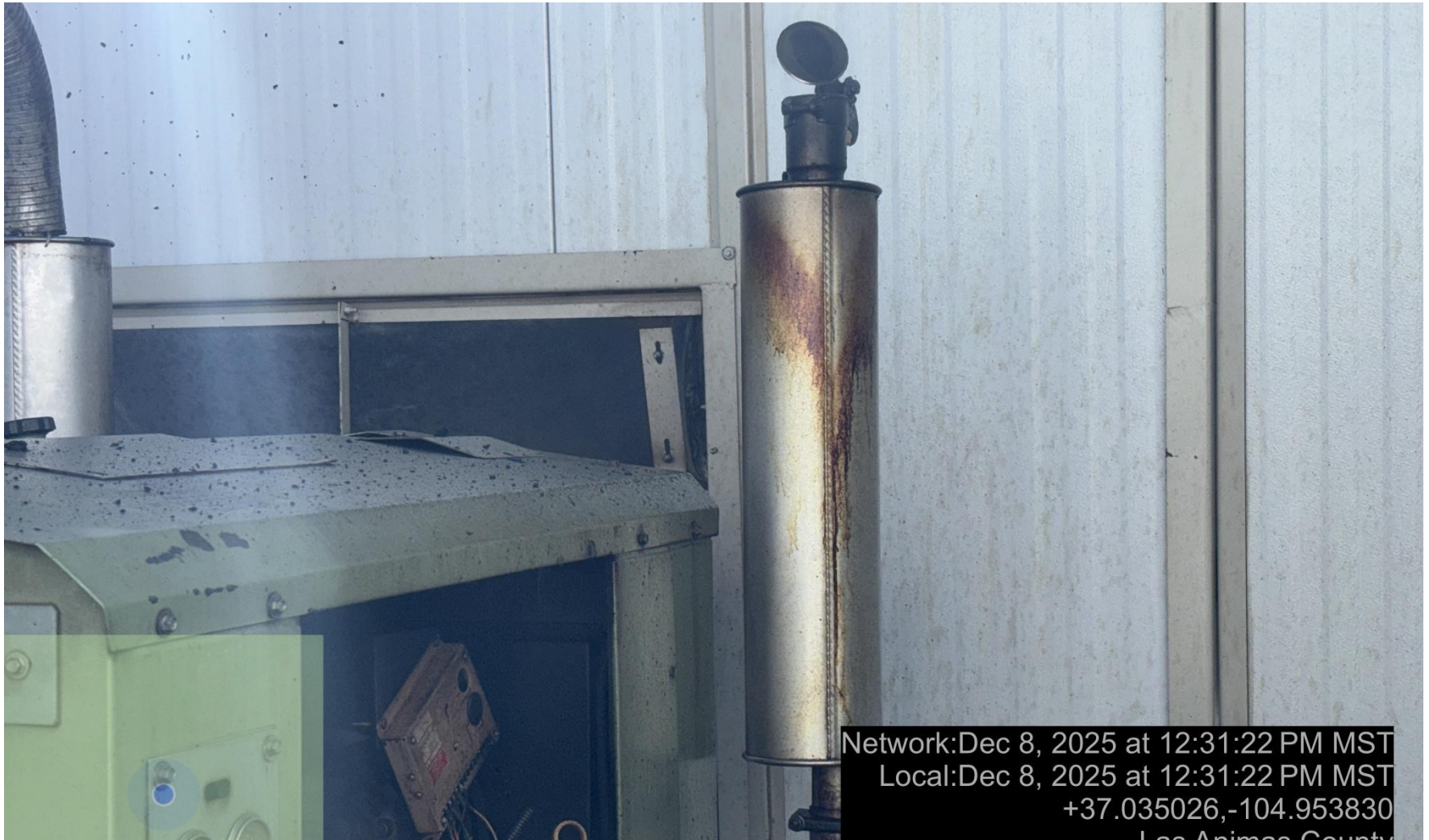
PHOTO 7: PRIME MOVER IS BLOWING OIL OUT OF EXHAUST PIPES. Securely fasten all valves, pipes, fittings, and Production Facilities to ensure good mechanical condition, inspect at regular intervals and maintain in good mechanical condition. Engineer, operate, and maintain equipment within the manufacturer's recommended specifications per Rule 608.e. CA DATE 12-9-2025.
