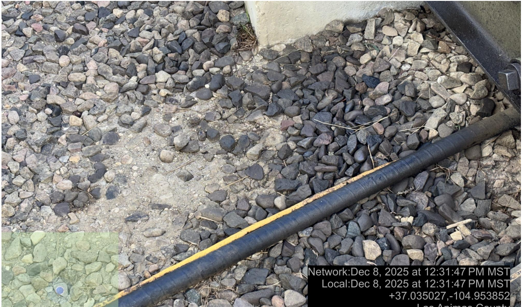
PHOTO 5: IMPACTED OIL NEAR PRIME MOVER SKID. Conduct maintenance on equipment, cleanup stained material and review self inspection processes. COMPLY WITH RULE 1002,(2).D. CA DATE 12-15-2025.
