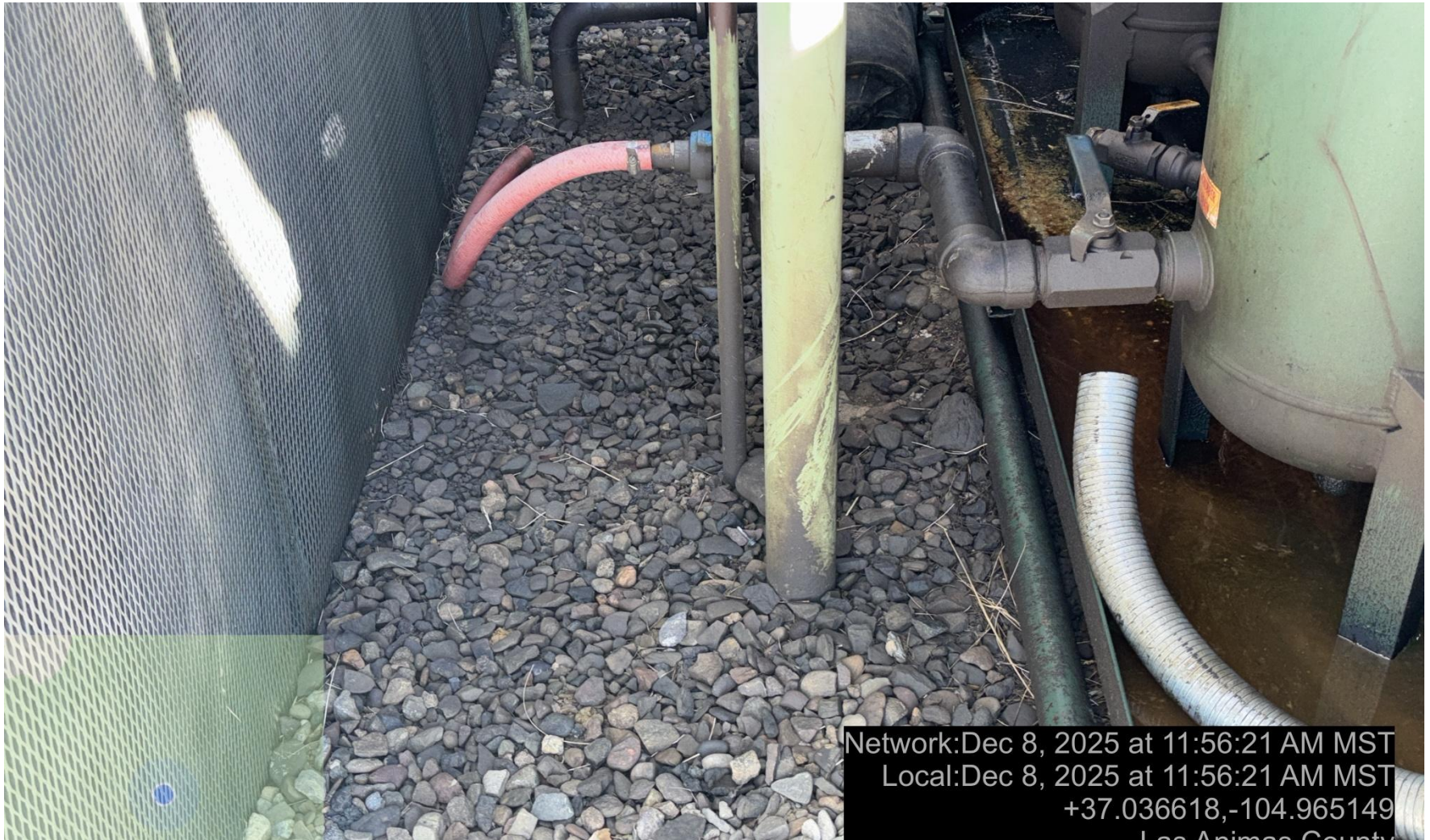
PHOTO 4: AREA OF IMPACTED SOIL NEAR COMPRESSOR SKID. Conduct maintenance on equipment, cleanup stained material and review self inspection processes. COMPLY WITH RULE 1002,(2).D. CA DATE 12-15-2025.
