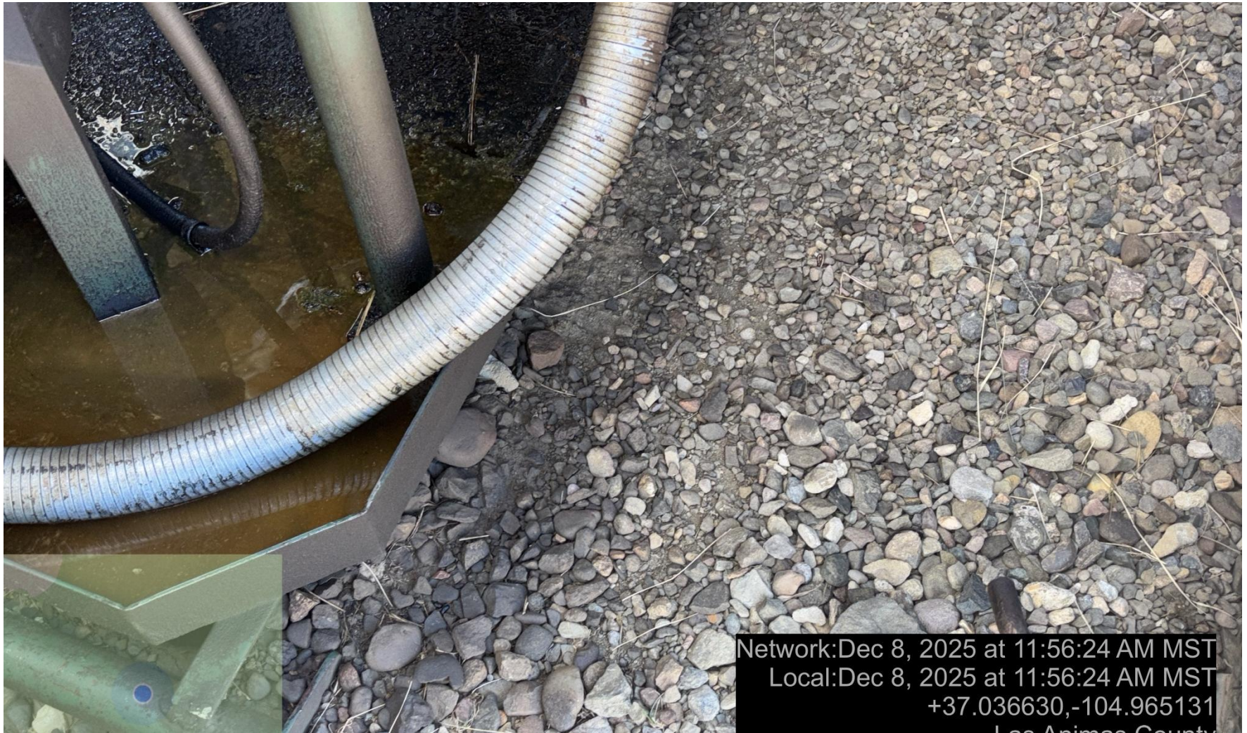
PHOTO 5: AREA OF IMPACTED SOIL NEAR COMPRESSOR SKID. Conduct maintenance on equipment, cleanup stained material and review self inspection processes. COMPLY WITH RULE 1002,(2).D. CA DATE 12-15-2025.
