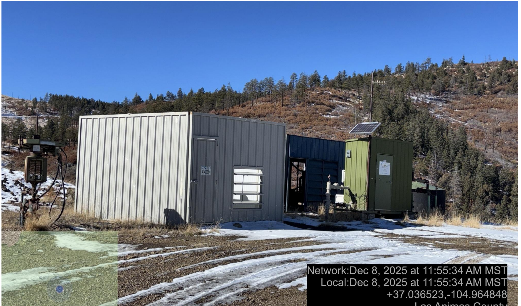
PHOTO 3: WELLHEAD AND EQUIPMENT.
