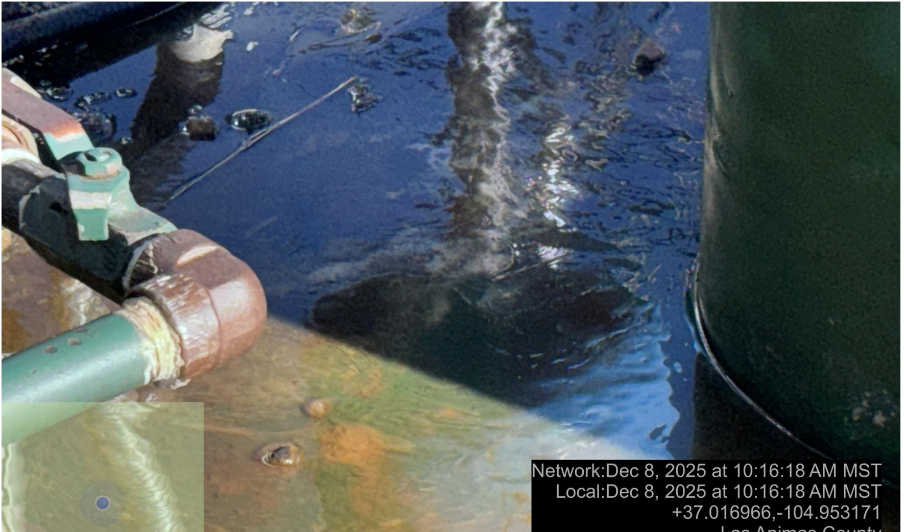
PHOTO 6: OILY FILM IN COMPRESSOR SKID. DRAIN OILY WASTE REPAIR ALL LEAKS AND REMOVE IMPACTED SOIL PER RULE 1002..(2).D & 1002.f.(2)B, Comply with general provisions of the oil and gas act for wildlife protection AND SB-181. CA DATE 12-9-2025.
