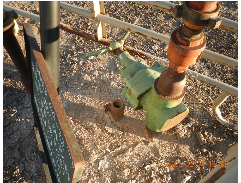
2. View of wellhead. Note Bradenhead valve missing plug.
