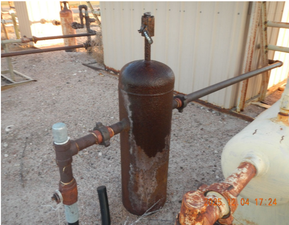
5. View of Dehydrator (Drip Bottle) on gas meter run inlet. Note visible moisture on bottle.
