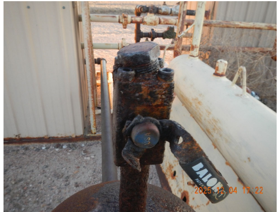
6. View of valve on Dehydrator (Drip Bottle). Valve will not full close and plug seat is cross threaded.
