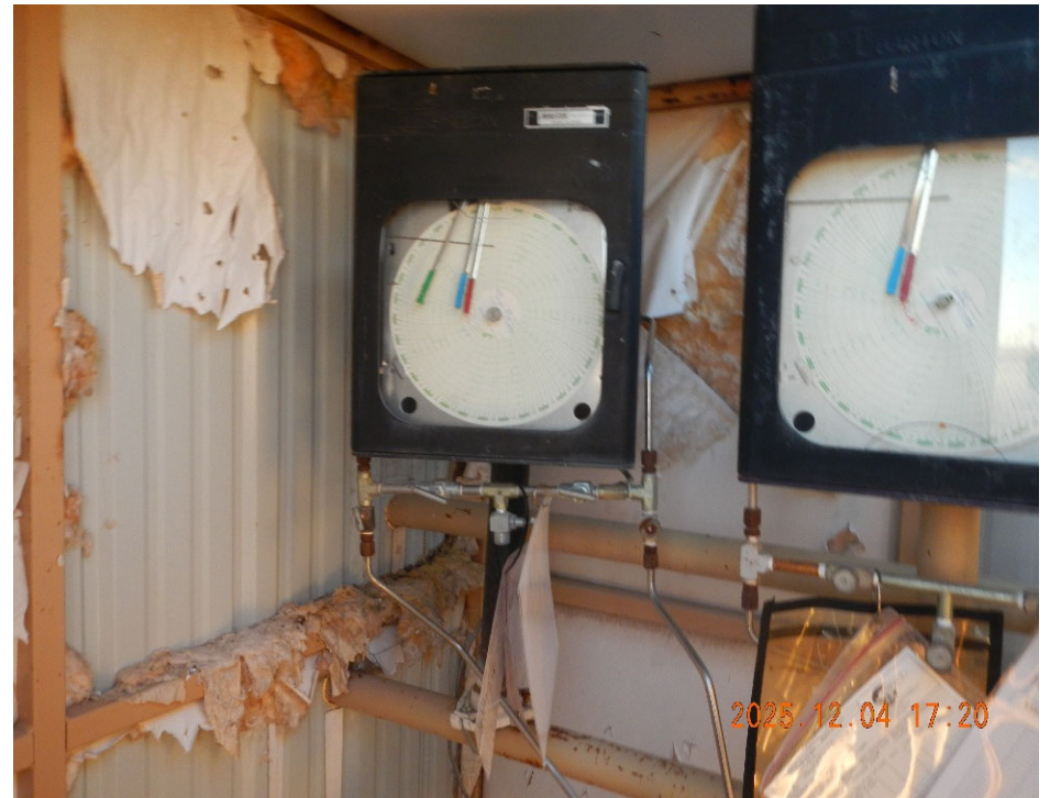
8. Gas meter inside meter shed.
