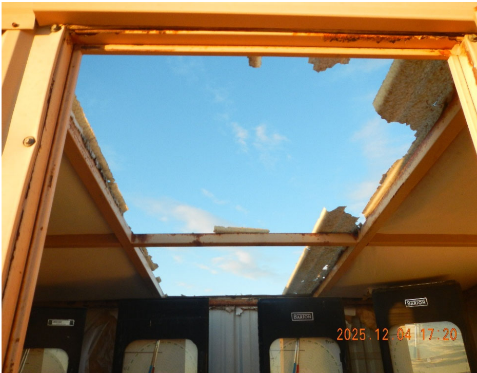
7. Damage to Meter Shed roof.
