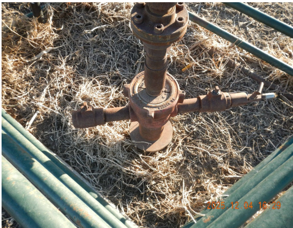
3. View of wellhead. Note Bradenhead not visible at surface.
