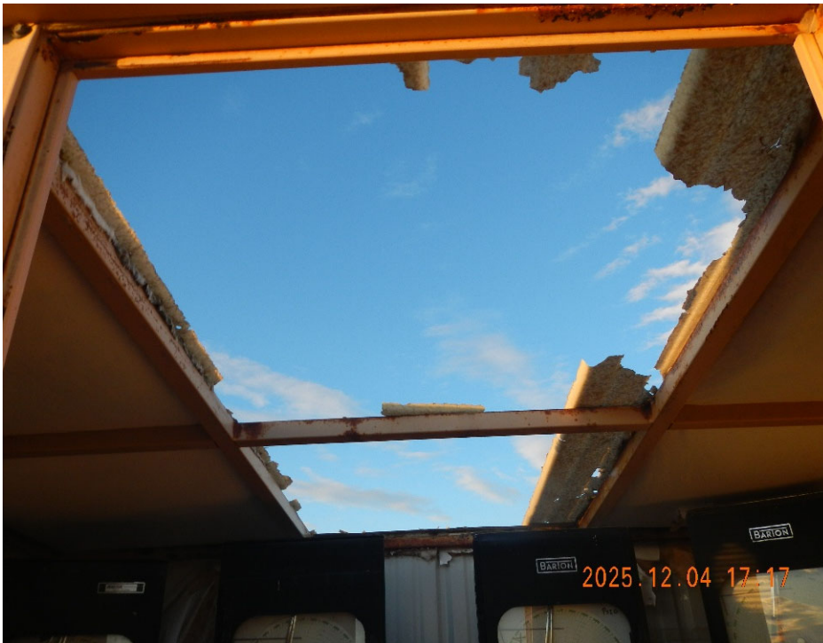
7. Damage to Meter Shed roof.
