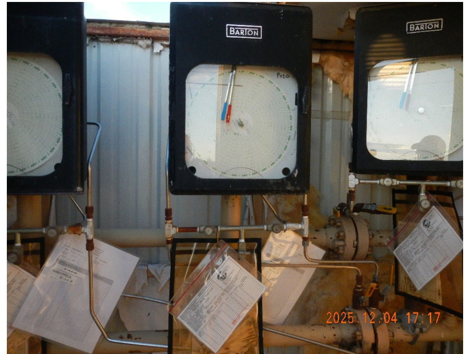
8. Gas meter inside meter shed.
