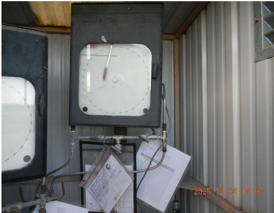
5. Gas Meter inside Meter Shed.
