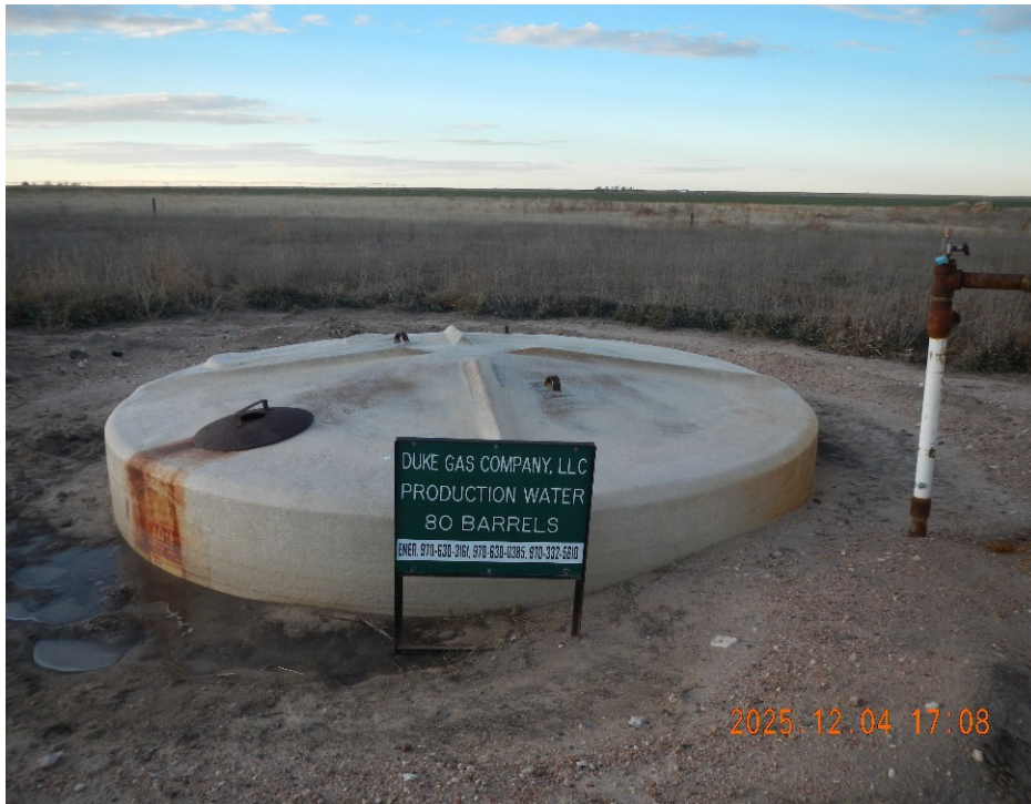
7. View of produced water tank at remote gathering location.
