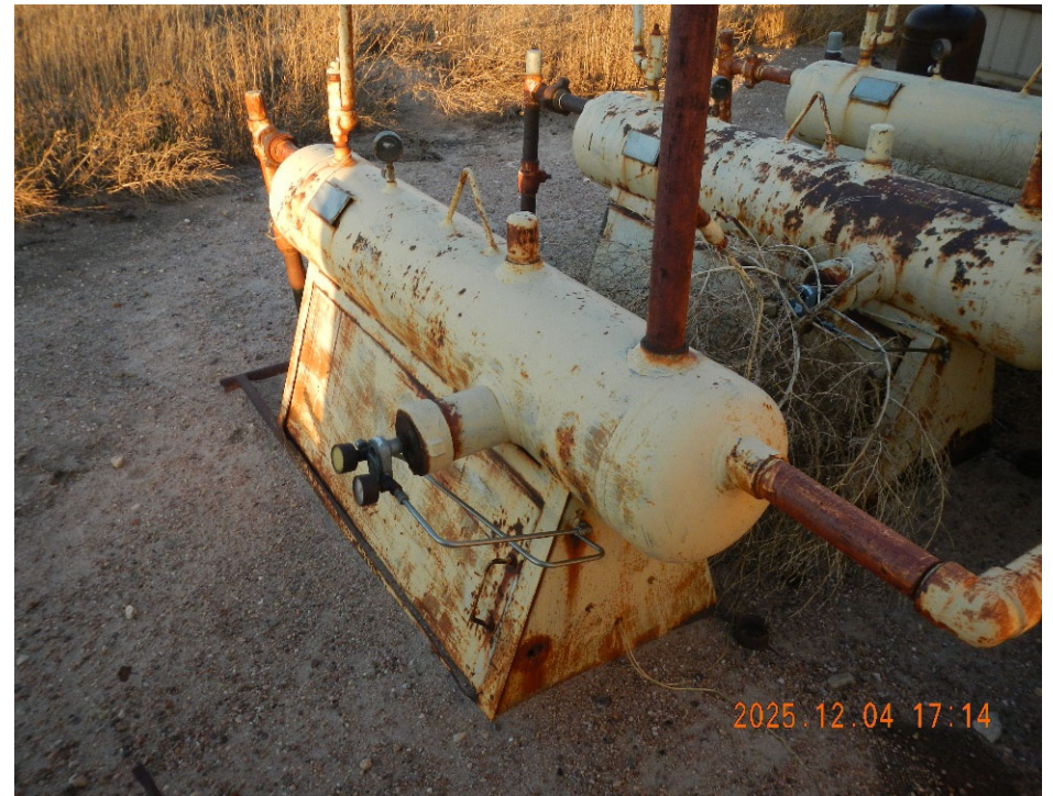
6. View of horizontal separator at gathering location.
