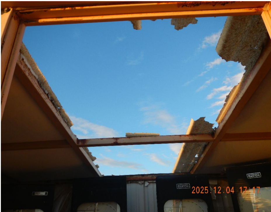
7. View of damaged gas meter Shed roof.
