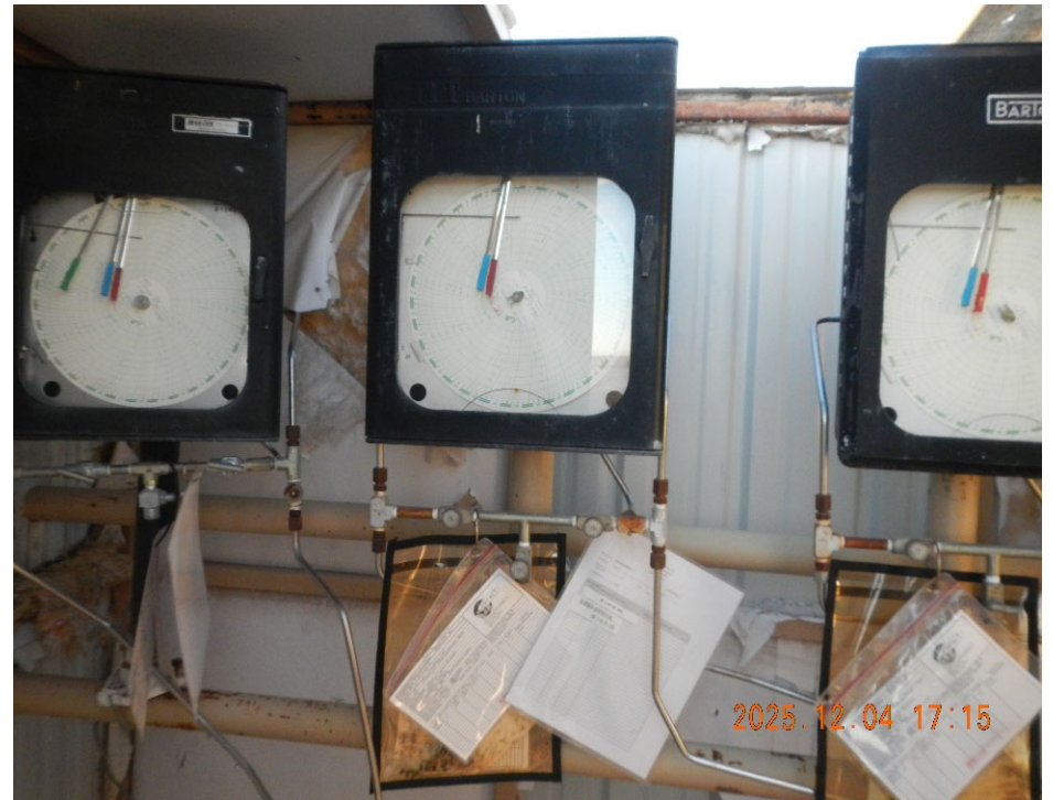
8. Gas meter inside meter shed.
