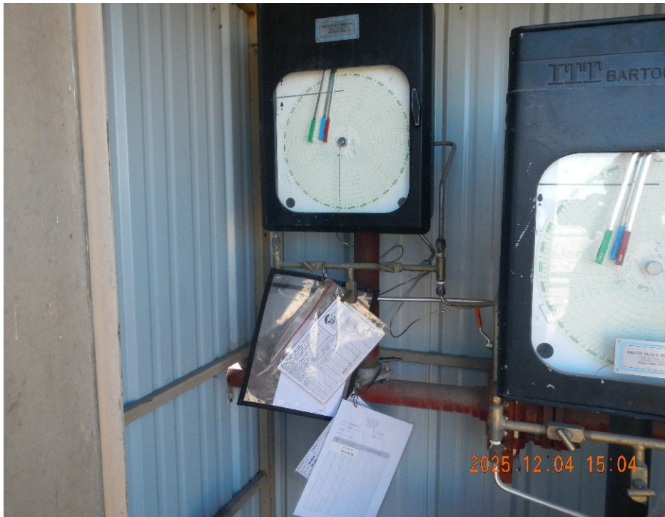
5. Gas Meter inside Meter Shed.
