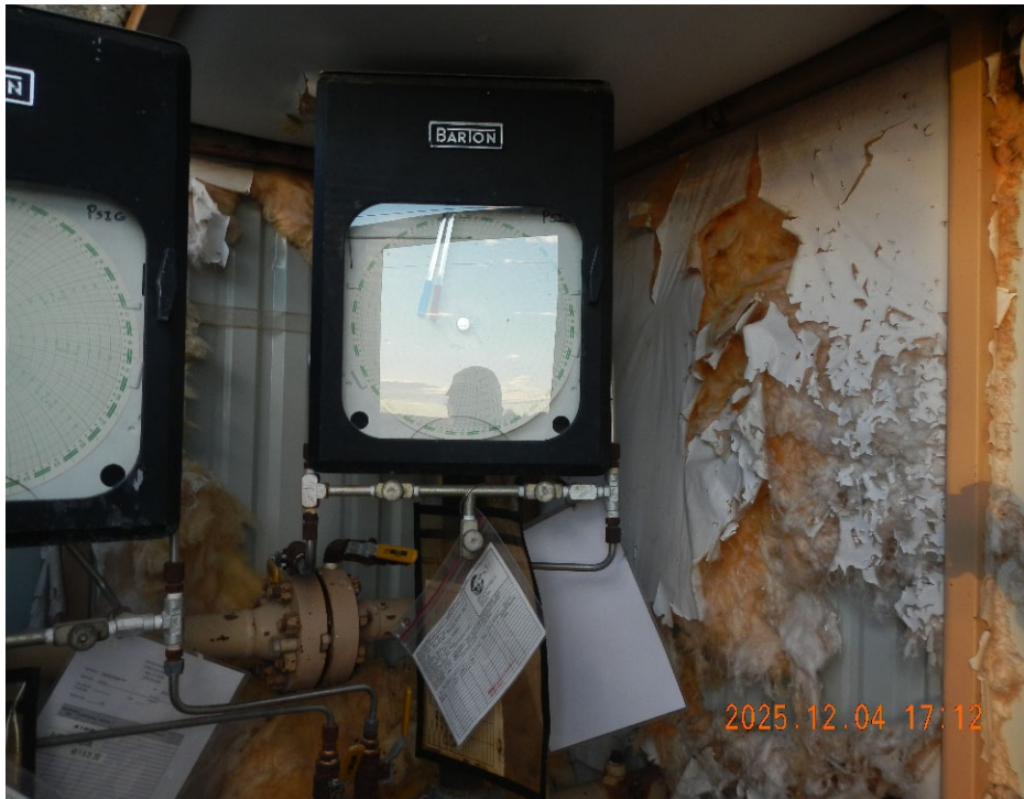
7. Gas Meter inside Meter Shed.
