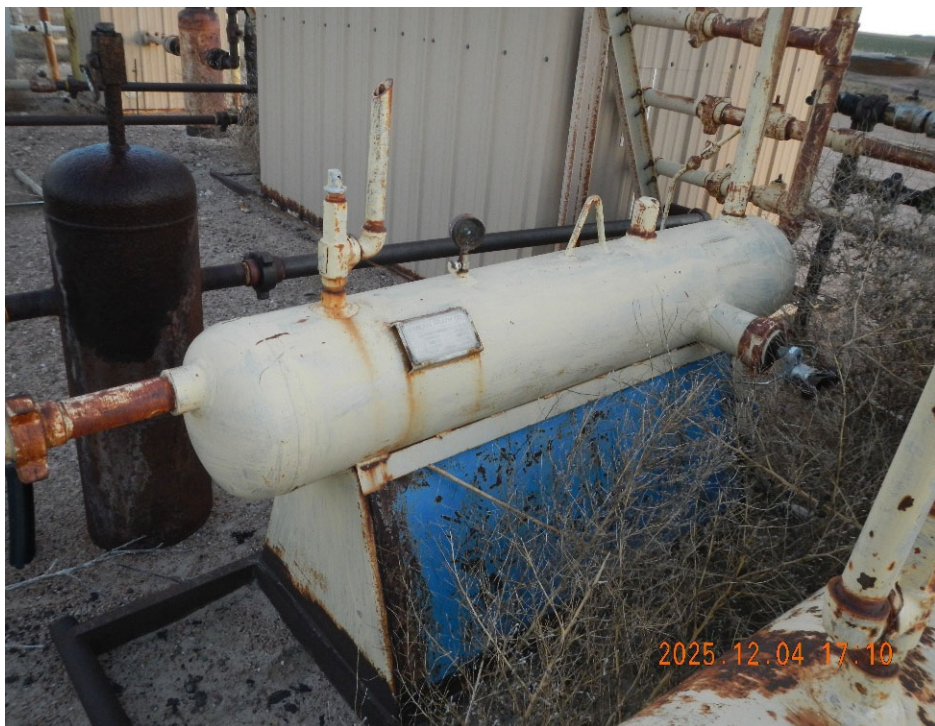
5. View of horizontal separator at remote gathering location.
