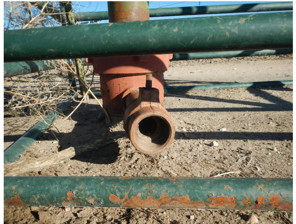
2. Bradenhead valve found open at time of inspection.
