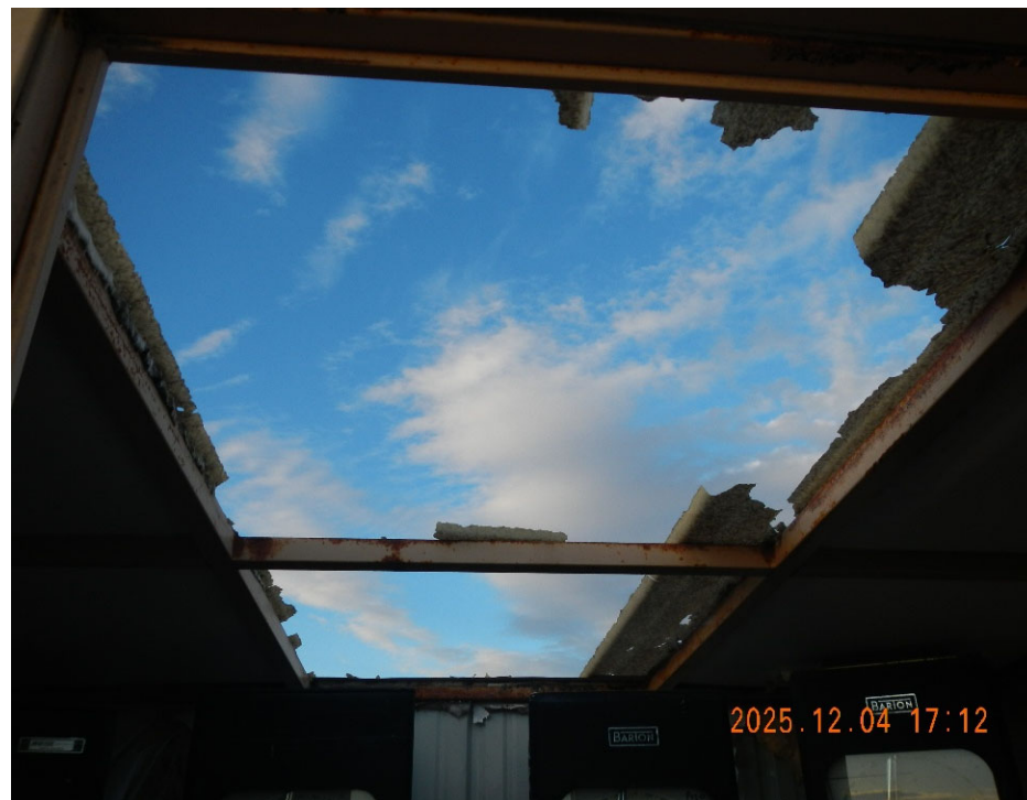
6. Damage to Meter Shed roof.
