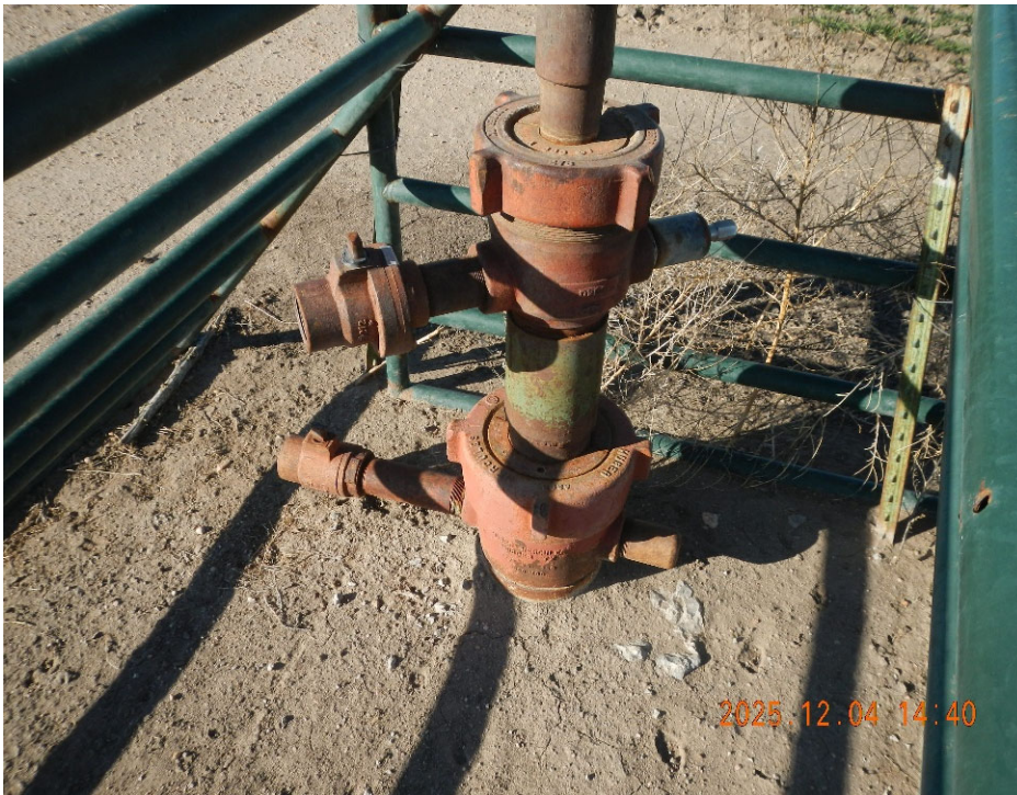
1. View of wellhead. Note both the casing valve and bradenhead valve are missing plugs.
