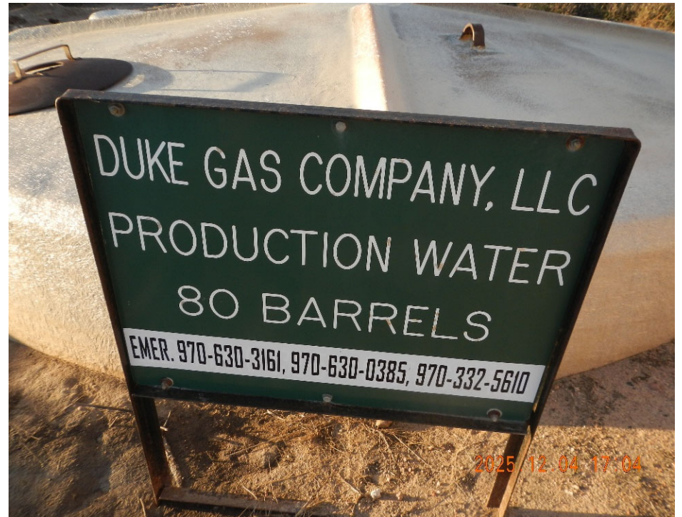
6. Tank sign missing NFPA label.
