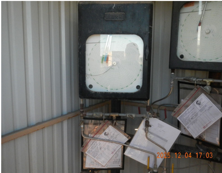
5. Gas Meter inside Meter Shed.
