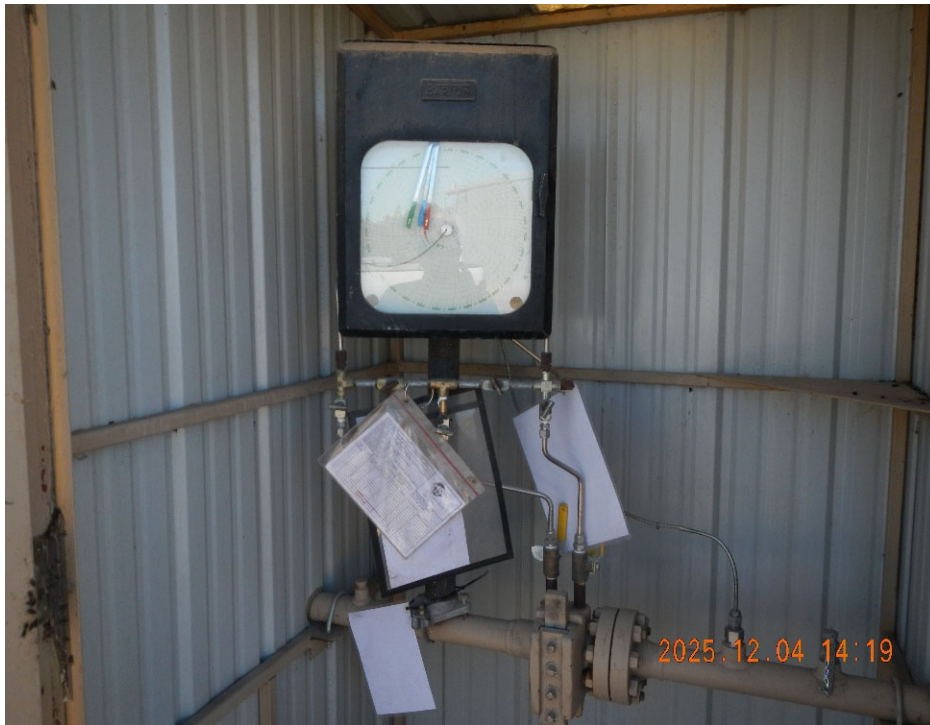
5. Gas Meter inside Meter Shed.
