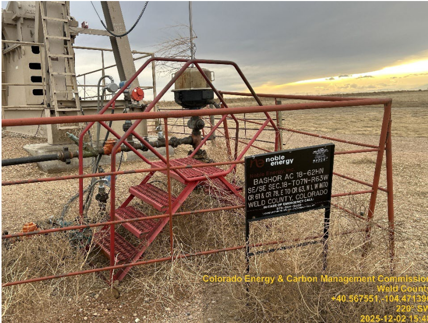
Photo #1 Bashor AC 18-62HN (123-35093) Wellsite Producing | PR
