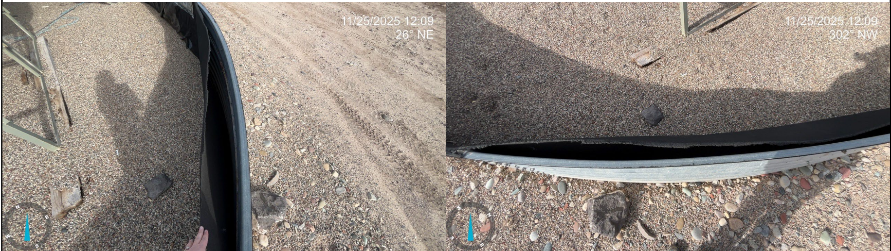
Photo 3: Photos showing the secondary containment liner at tank equipment is no longer sufficiently impervious. Comply with Rile 603.o.
