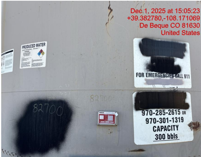
Tank Labels Missing Required Information – Photo #01783
