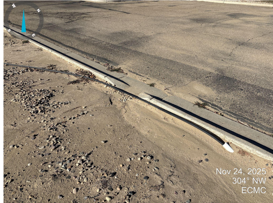
Photo 4. Photo taken on the north side of the location. It appears that sediment is leaving the location through this drain in the curb.
