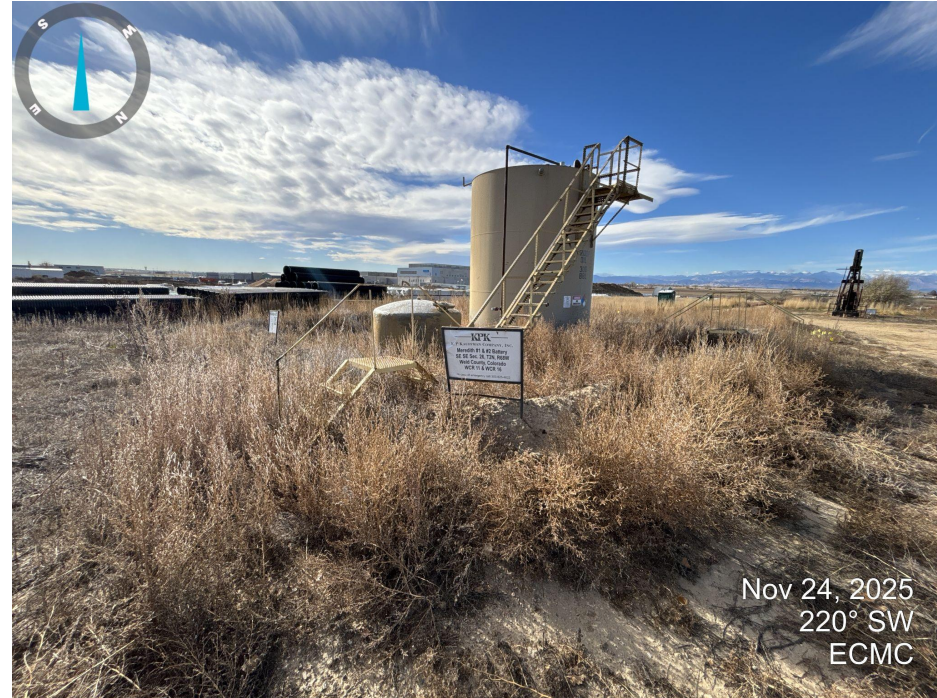
Photo 2. Looking south at the tank battery located to the east of the wellhead. Undesirable weeds such as kochia are unmanaged on location and touching equipment.
