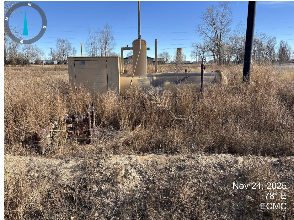
Photo 4. Photo taken at the separator on the tank battery. Undesirable weeds are unmanaged on location. Weeds are touching equipment.
