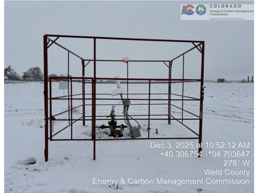
Photo 2 well head and equipment
