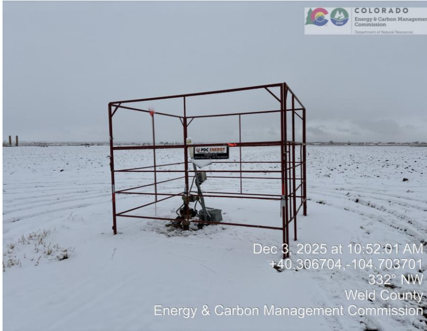
Photo 1 well head and equipment
