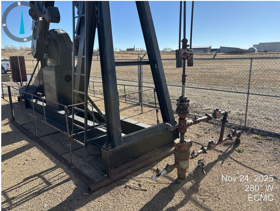
Photo 3. Picture taken at the wellhead.
