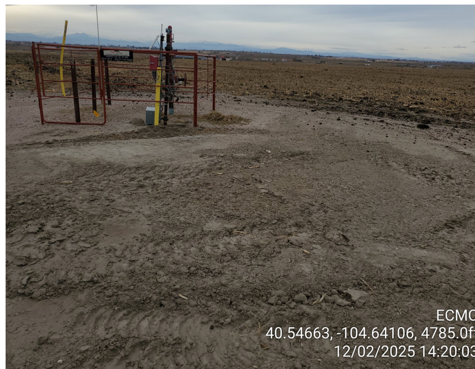
Location of Harper USX EE27-23D, which is plugged and buried; Harper USX EE27-15D is in background
