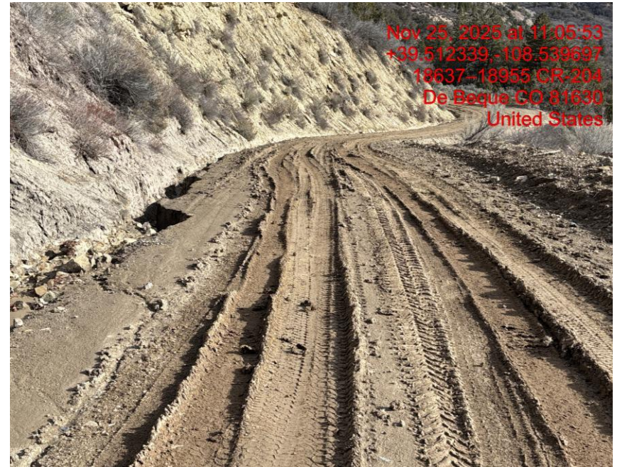
Lack of Stabilization/Insufficient Erosion Controls on Lease Road – Photo #01774
