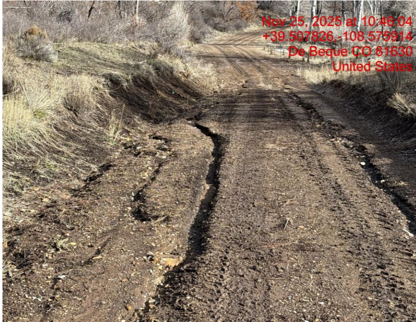
Insufficient Erosion Controls on Lease Road – Photo #01754
