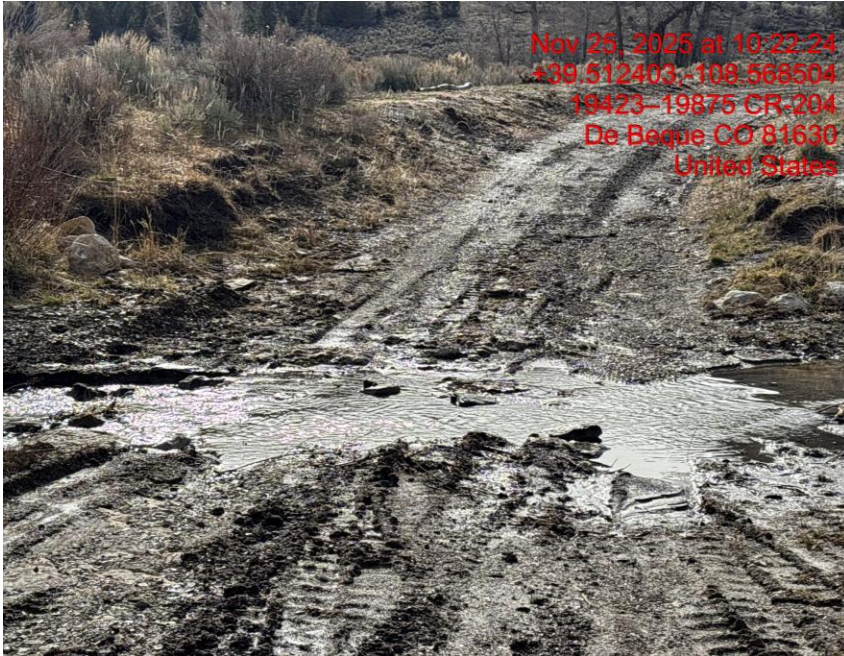
No BMPs or Erosion Controls at Stream Crossing – Photo #01731
