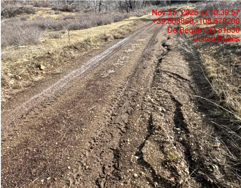
Insufficient Erosion Controls on Lease Road – Photo #01744
