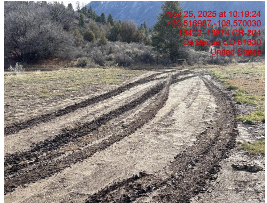
Lack of Stabilization/Insufficient Tracking BMPs – Photo #01729
