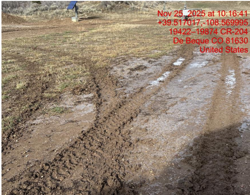
Lack of Stabilization – Photo #01724
