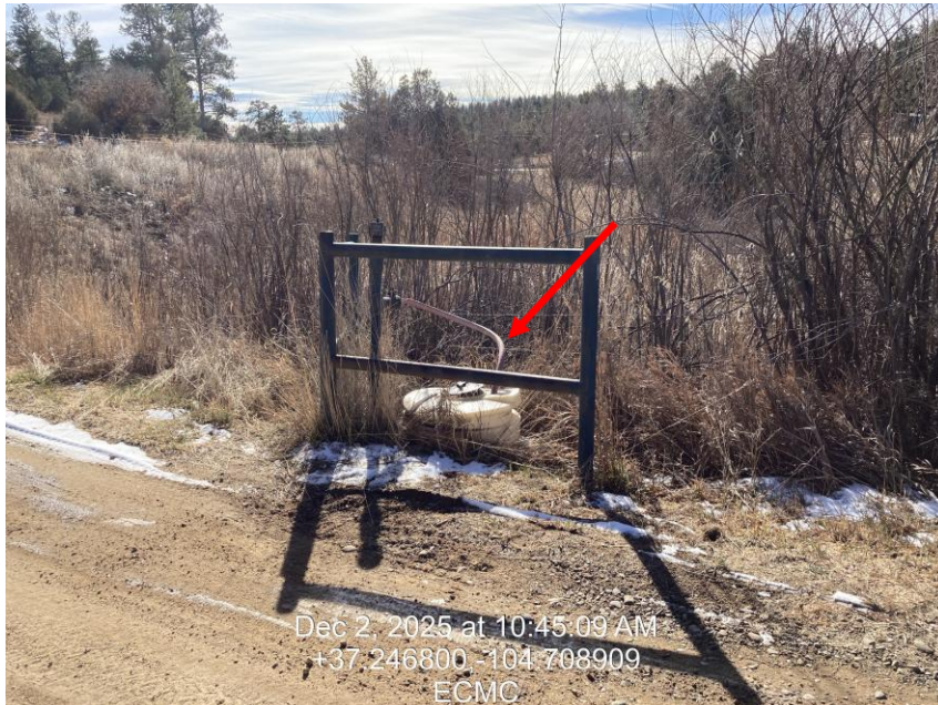
Photo 7 – Drip near county road intersection.
