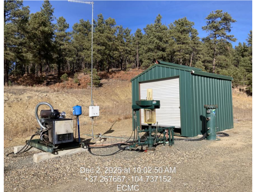
Photo 6 – TR wellhead API: 05-071-08520
