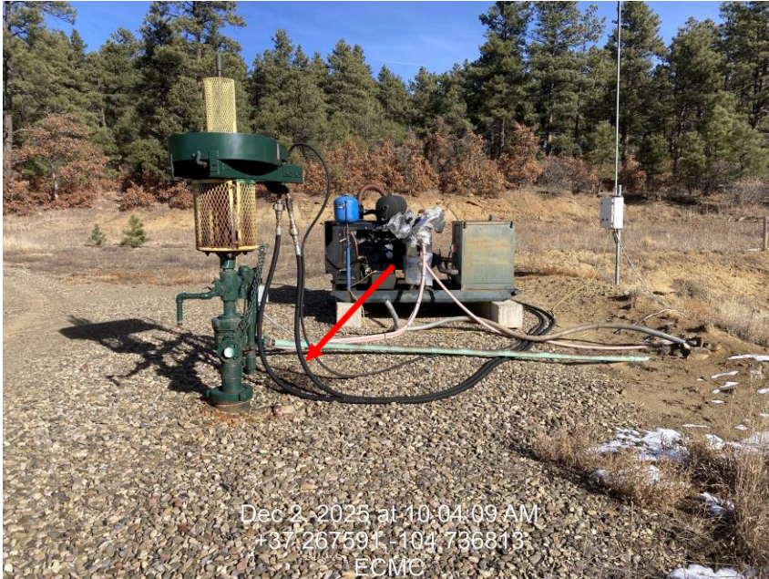
Photo 5 – Stained soils at base of KV wellhead
