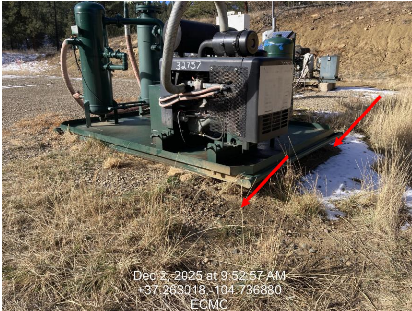
Photo 5 – Stained soils at base of skid.
