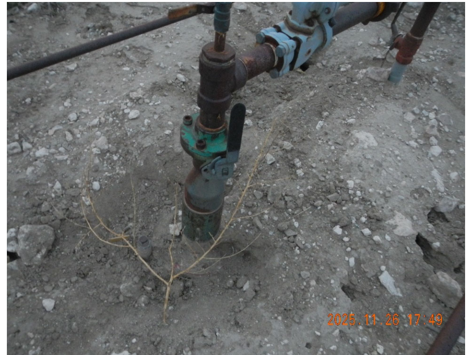
2. View of wellhead. Bradenhead visible at surface.
