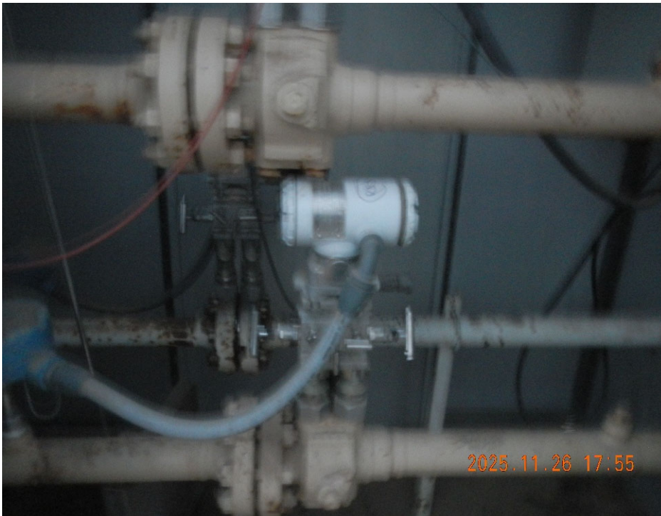
5. Gas Meter inside Meter Shed.
