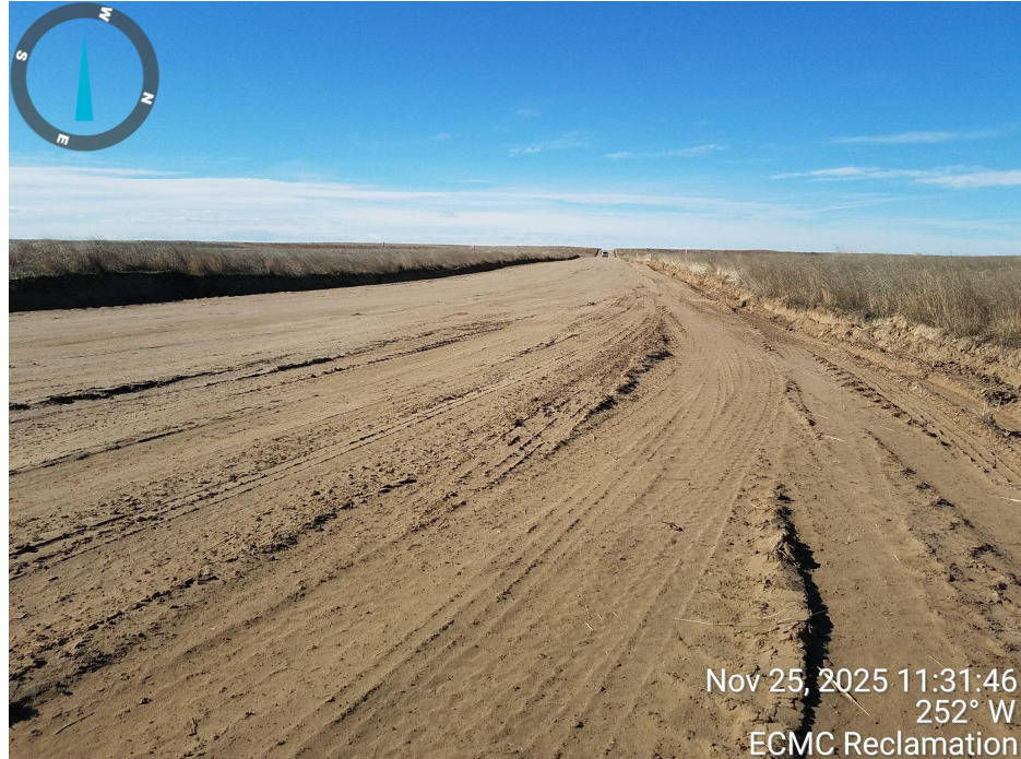
Photo 2. Photo taken from the entrance to location, facing West. Photo illustrates the Operator salvaged topsoil from the access road and is being stored on location.
