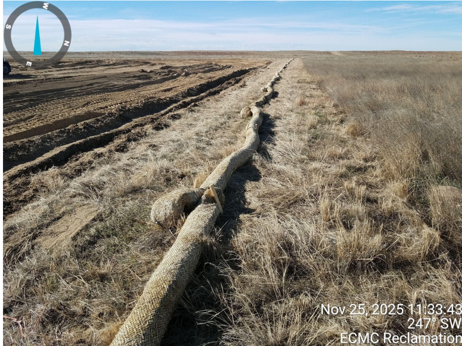
Photo 4. Photo taken from the northwestern perimeter of location, facing West. Photo illustrates the Operator installed a perimeter stormwater BMP around the entire perimeter of the location. However, the stormwater BMP (straw wattle) was not properly installed per good engineering practices.
