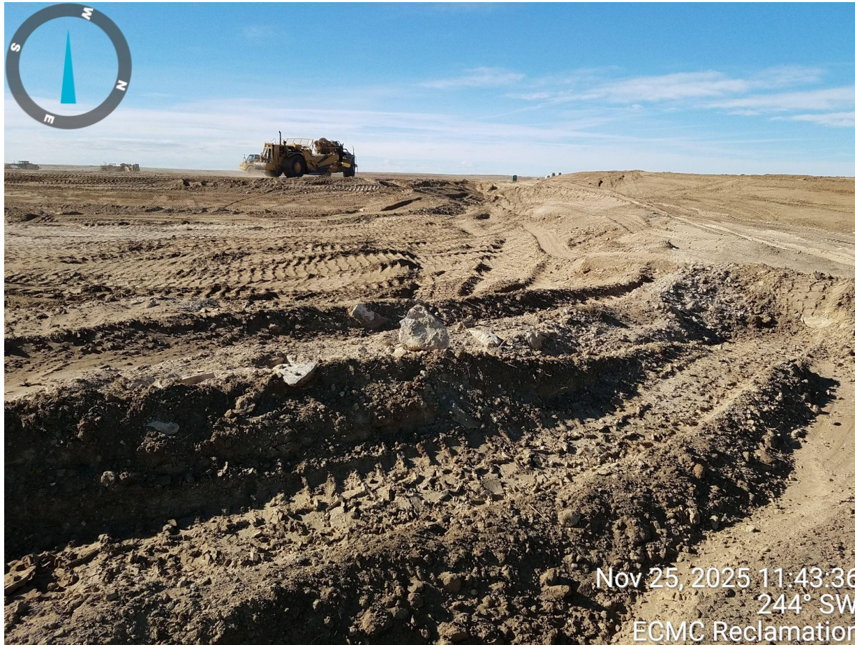
Photo 9. Photo taken from the northeastern location, facing West. Photo illustrates the Operator has completed topsoil salvage operations and is leveling out (cut/fill) the location.
