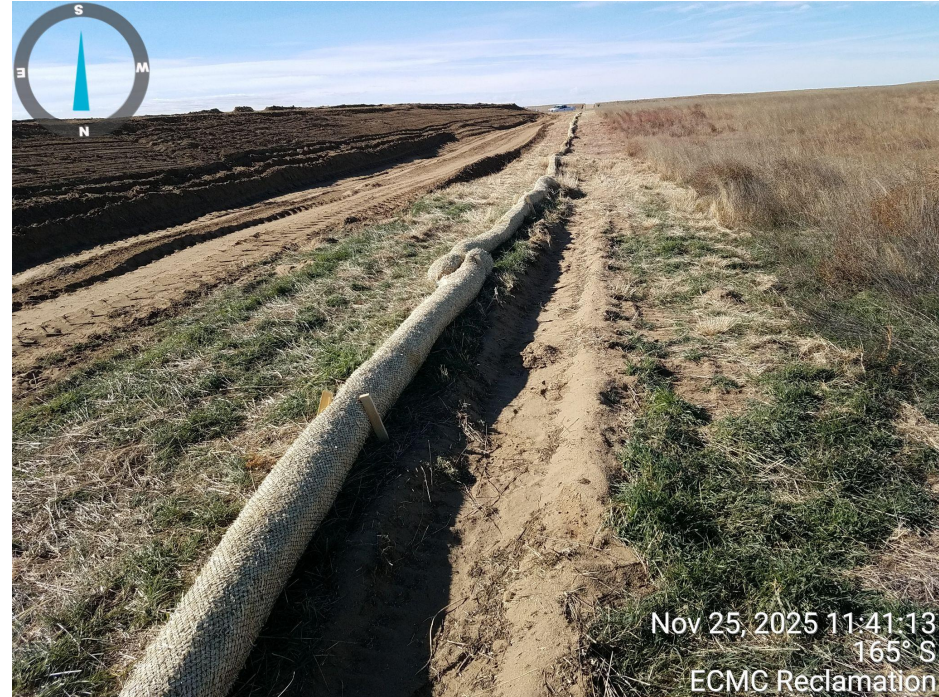
Photo 7. Photo taken from the northern perimeter of location, facing West. Photo illustrates a section of the stormwater BMP (straw wattle) illustrating the BMP has not been trenched in per good engineering practices. It appears that a trench was installed, yet the straw wattle was not placed within the trench. Note- the trench may be too deep for the straw wattle.
