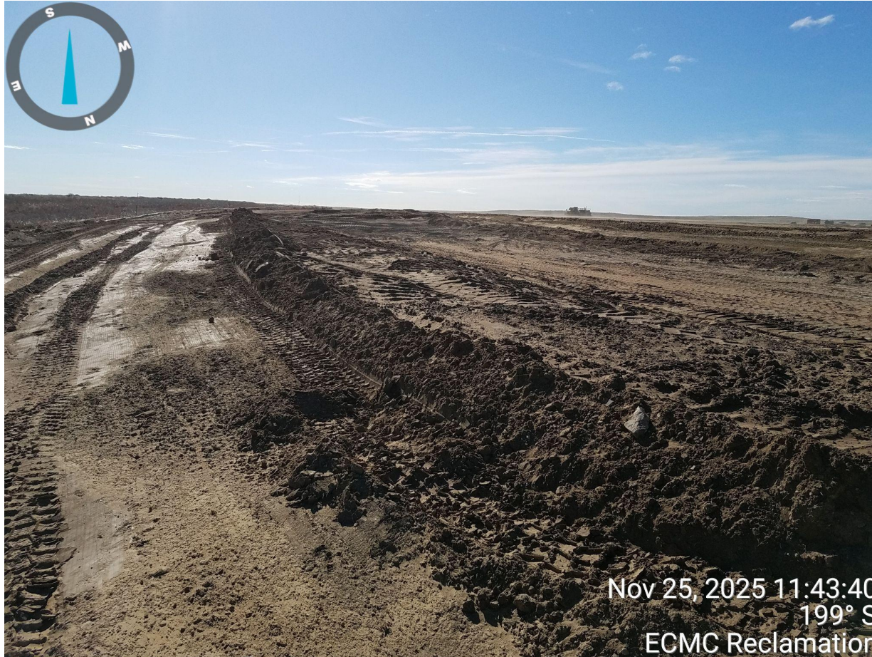
Photo 8. Photo taken from the northeastern location, facing South. Photo illustrates the detention pond is under construction and remains in-process.
