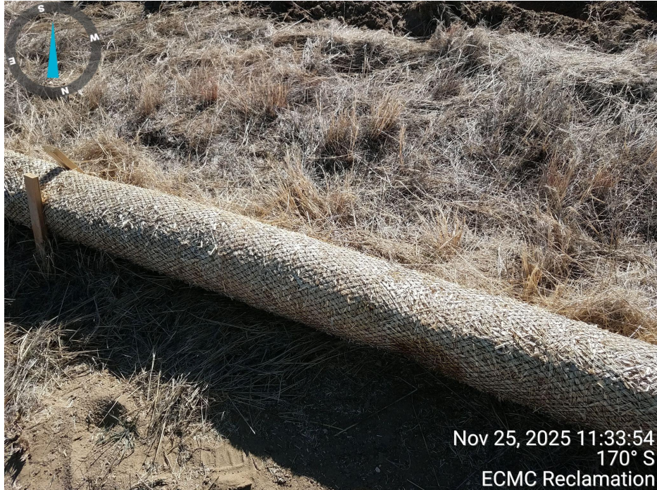
Photo 5. Close up photo taken from a section of the stormwater BMP (straw wattle) illustrating the BMP has not been trenched in per good engineering practices.
