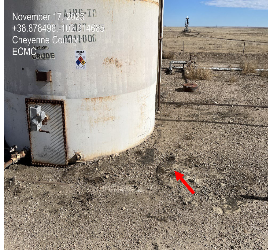
Photo 4. Oily impacts around base of the tank.
