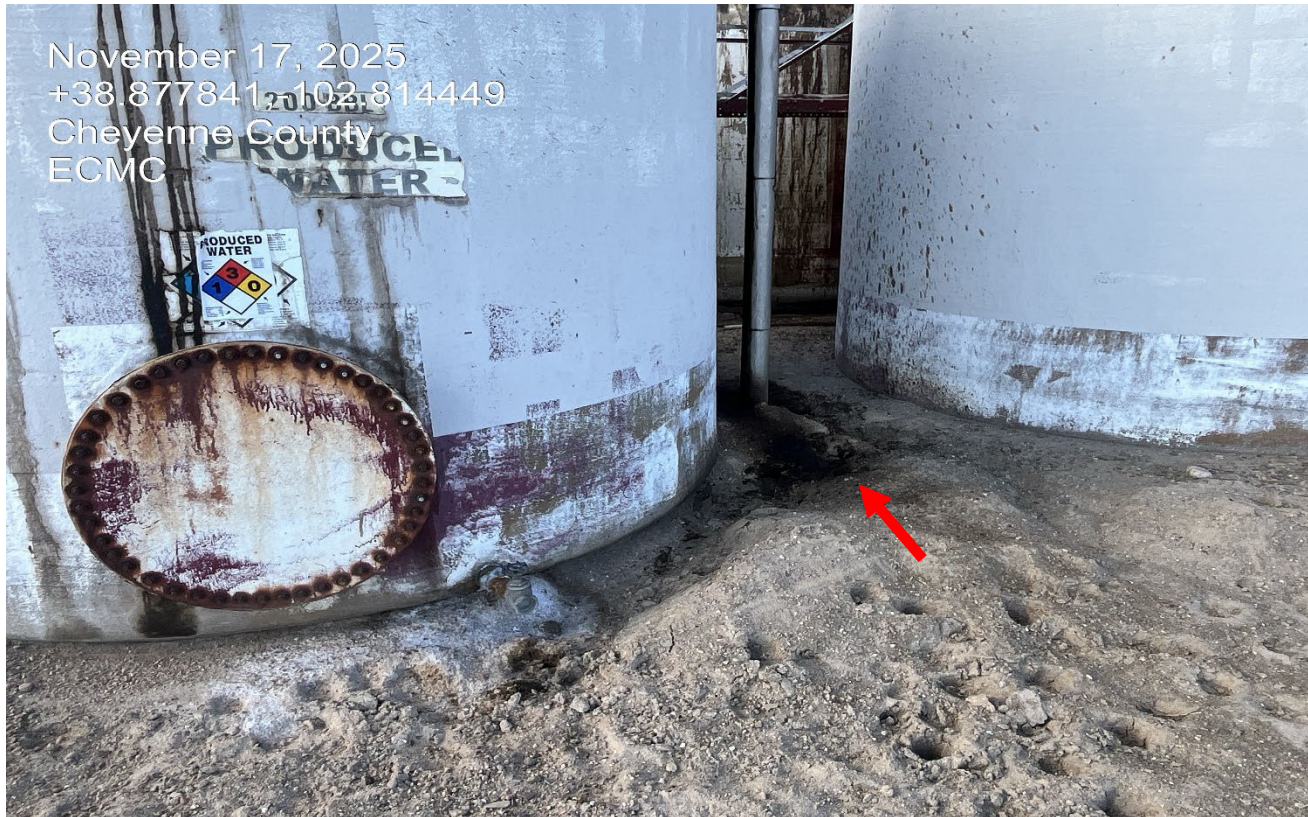
Photo 7. There are still impacts and leaks occurring at the base of the tank at the south side of the location.
