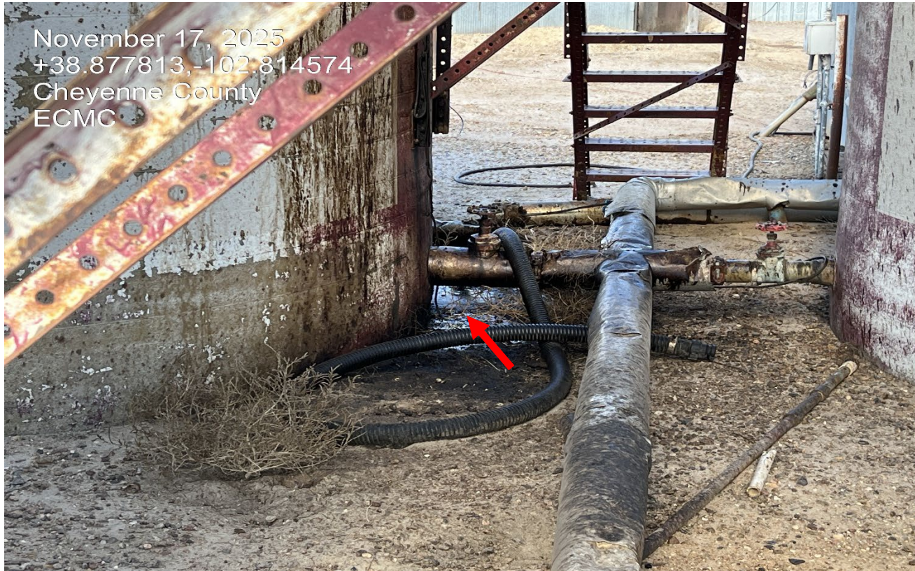
Photo 8. There are still impacts and leaks occurring at the base of the tank at the south side of the location.
