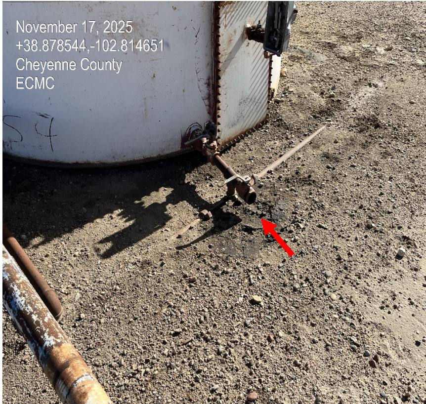
Photo 3. Oily impacts at pipe outlet.
