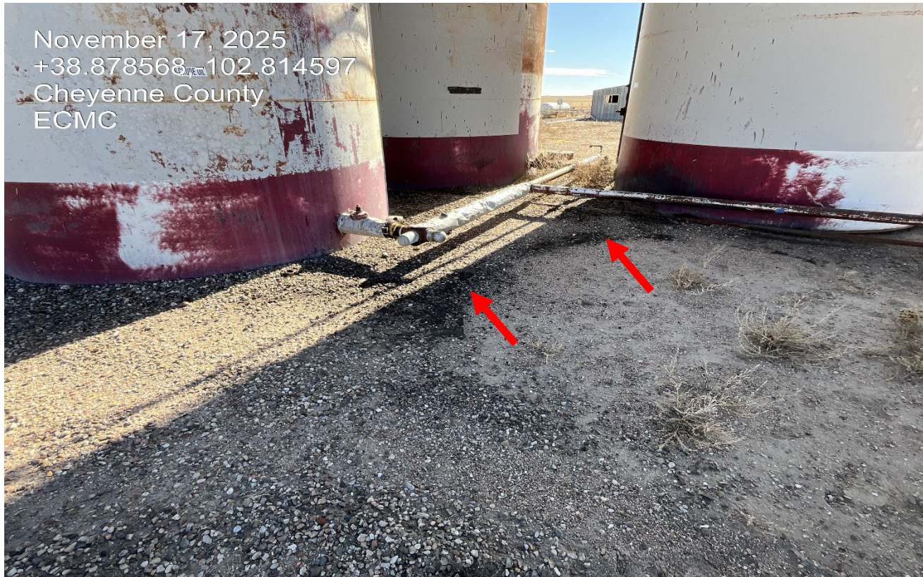
Photo 2. There are still oily impacted material around the tanks that have not been cleaned up.
