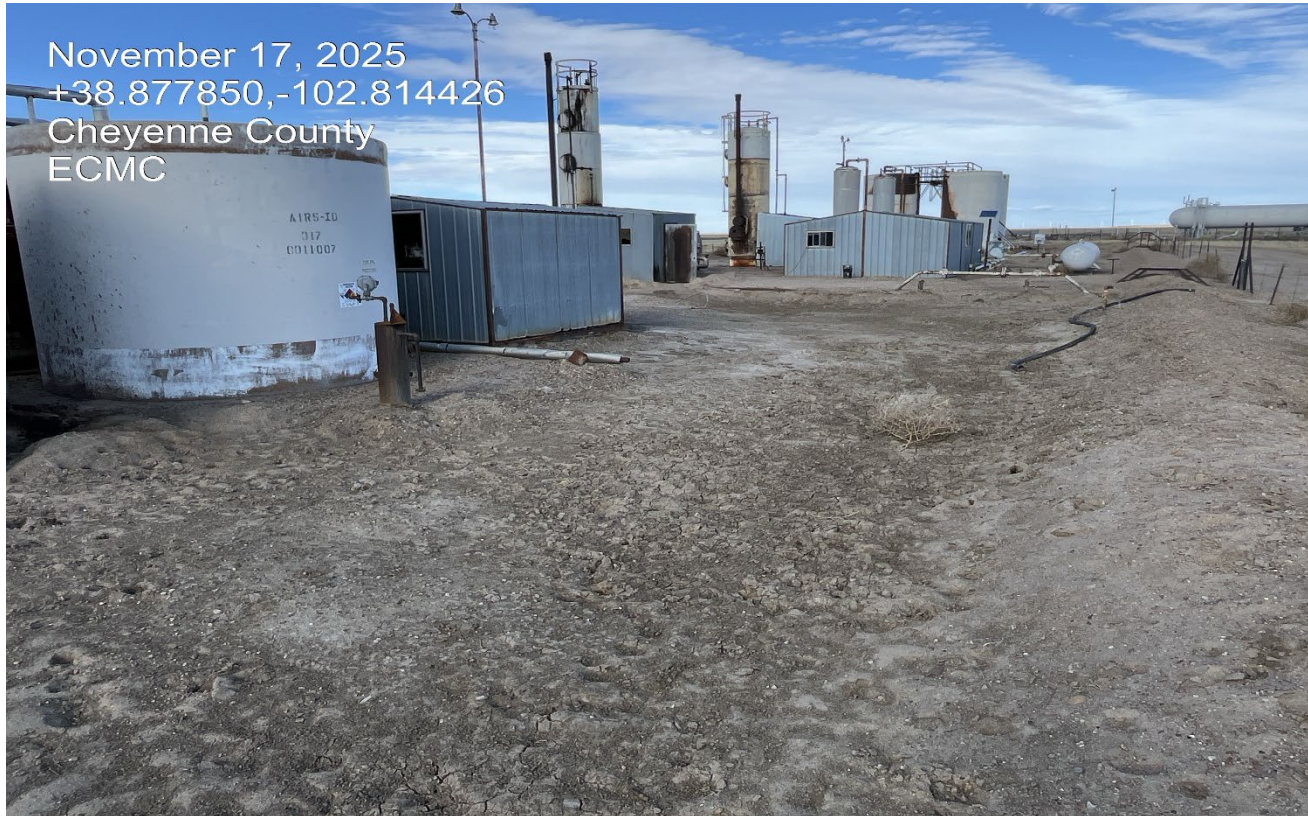
Photo 6. Facing west toward the area where new and additional spill recently occurred.
