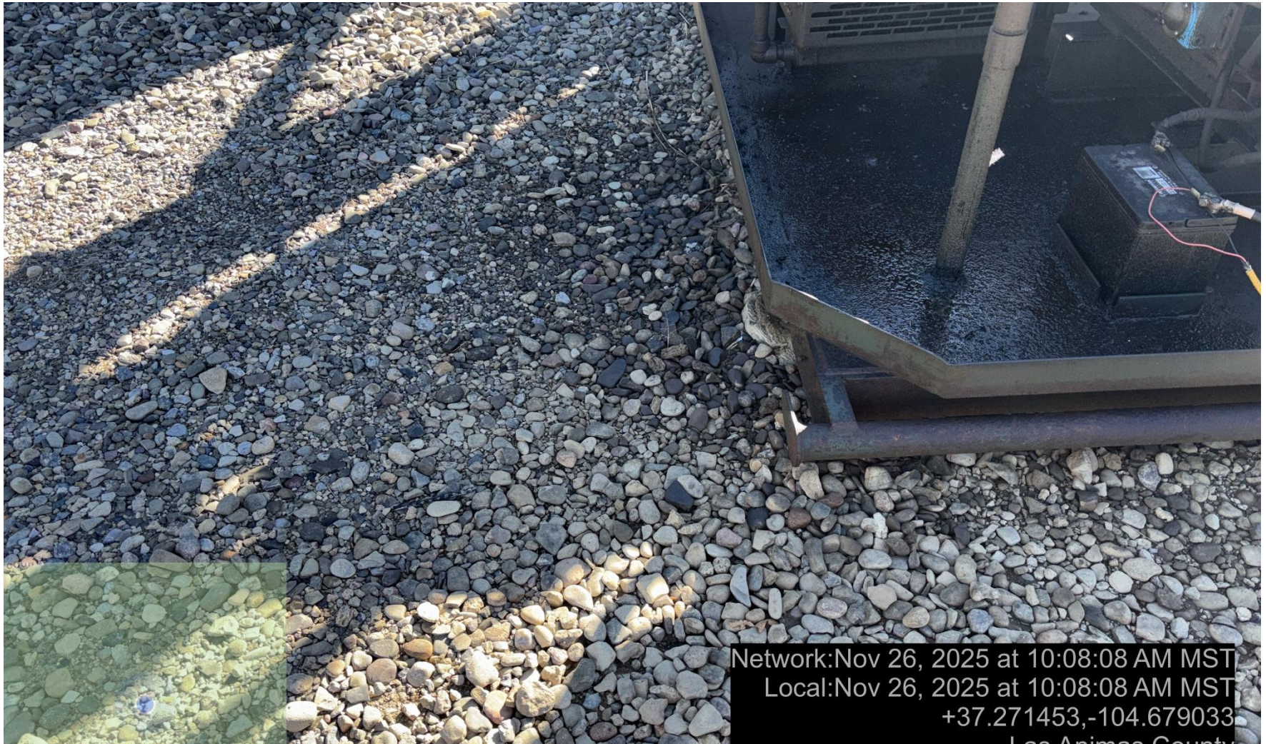
PHOTO 5: AREA OF IMPACTED SOIL AROUND COMPRESSOR SKID. Conduct maintenance on equipment, cleanup stained material and review self inspection processes. COMPLY WITH RULE 1002,(2).D. CA DATE 12-3-2025.
