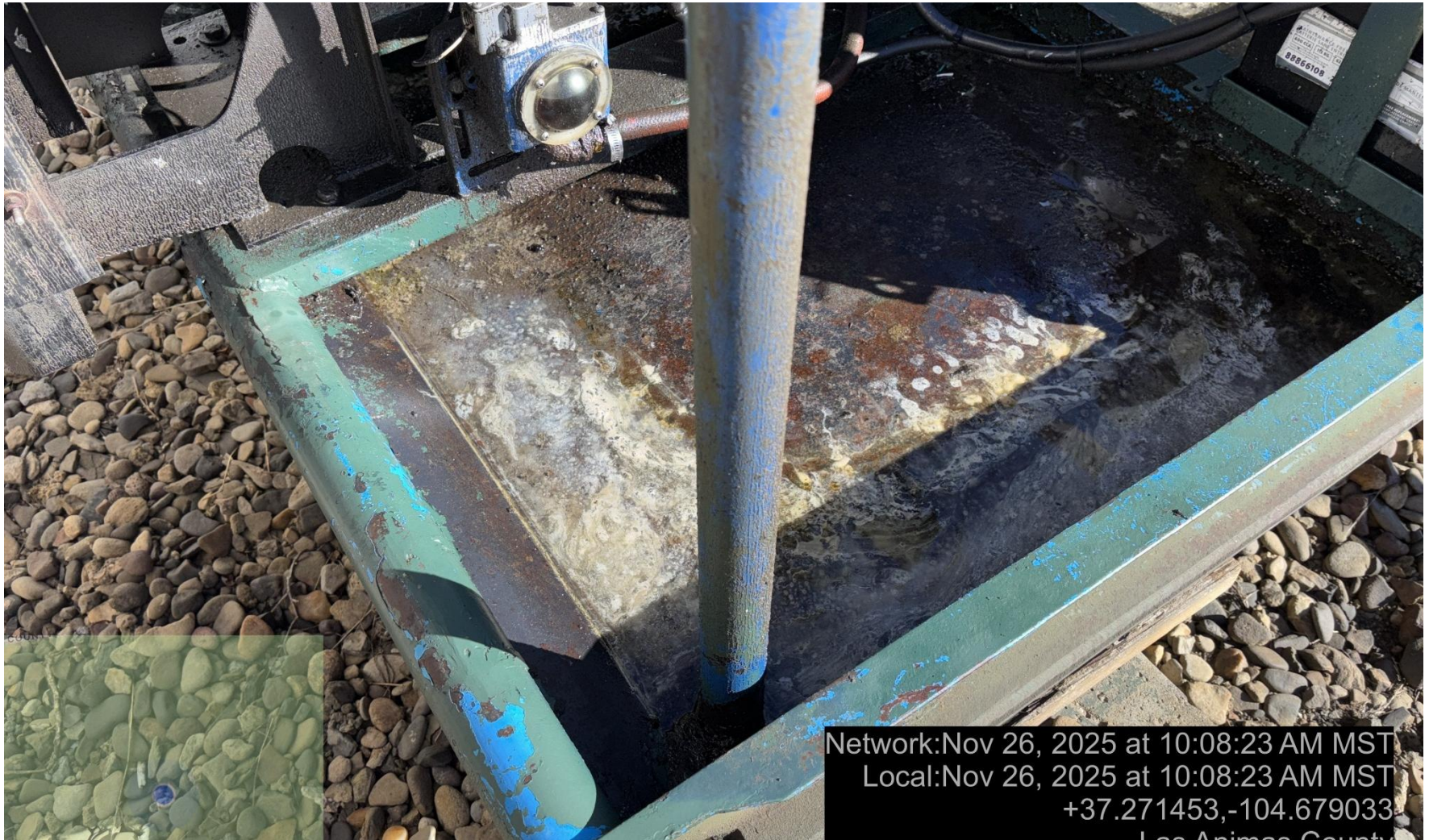
PHOTO 7: OILY WASTE IN ORIG. WELL PRIME MOVER SKID. DRAIN OILY WASTE REPAIR ALL LEAKS AND REMOVE IMPACTED SOIL PER RULE 1002..(2).D & 1002.f.(2)B, Comply with general provisions of the oil and gas act for wildlife protection AND SB-181. CA DATE 11-27-2025.
