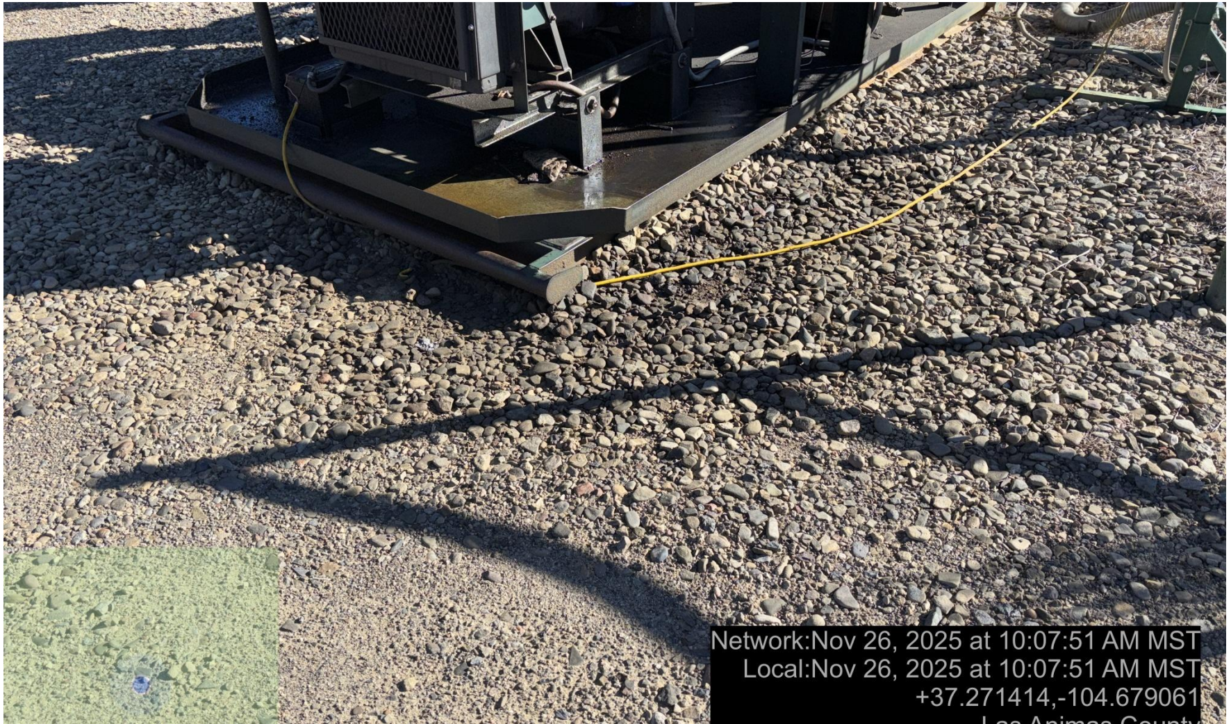
PHOTO 4: AREA OF IMPACTED SOIL AROUND COMPRESSOR SKID. Conduct maintenance on equipment, cleanup stained material and review self inspection processes. COMPLY WITH RULE 1002,(2).D. CA DATE 12-3-2025.
