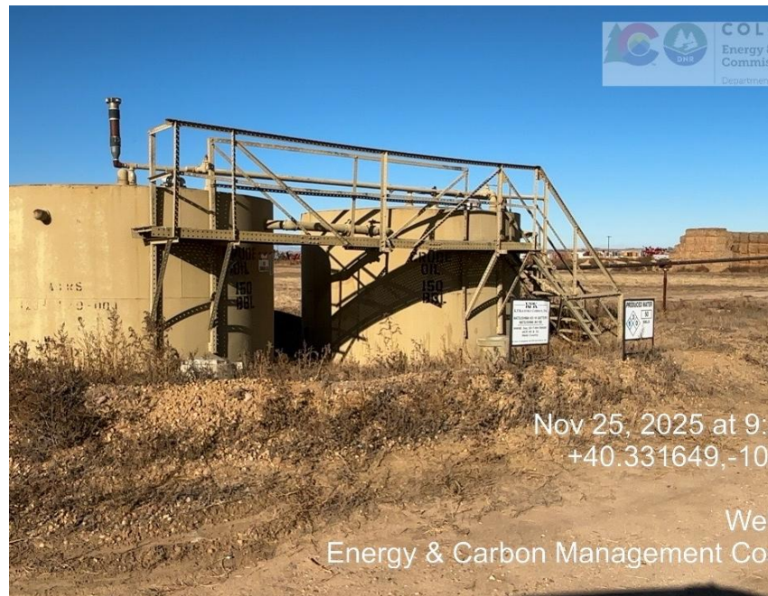
Photo 4 tank battery and equipment
