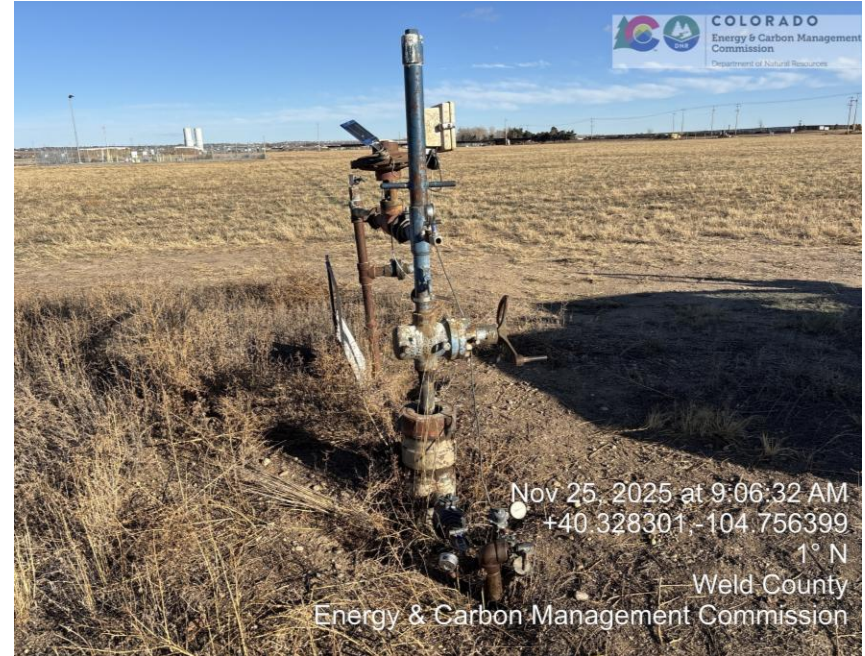
Photo 2 well head and equipment
