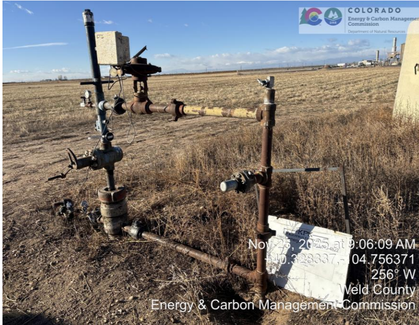
Photo 1 well head and equipment
