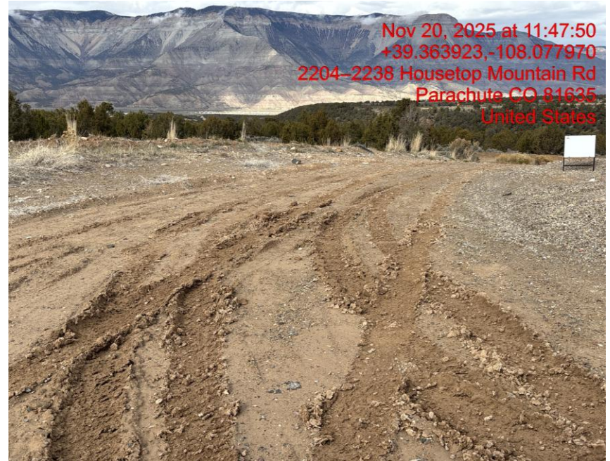
Insufficient Tracking BMPs – Photo #01643
