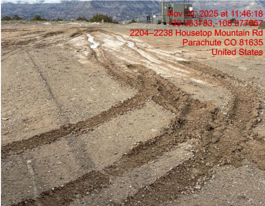
Lack of Stabilization – Photo #01641
