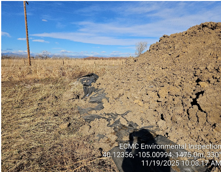
Photo 15 – Soil stockpile. Stormwater BMPs missing/inadequate.
