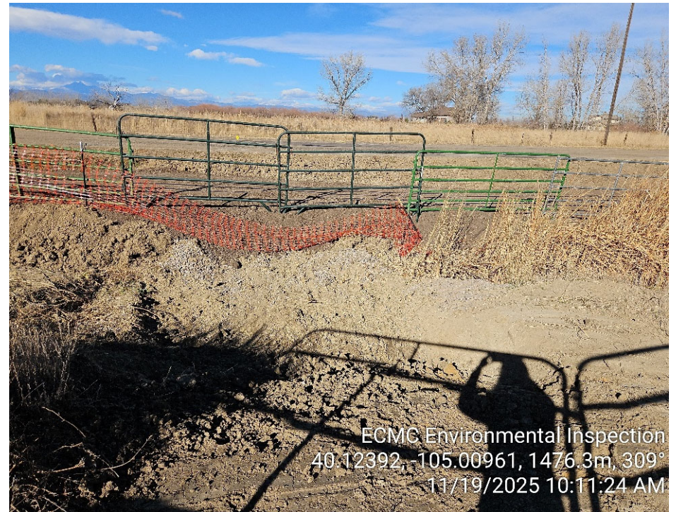
Photo 6 - Open excavation. No groundwater currently present. Excavation appears to have been partially backfilled.
