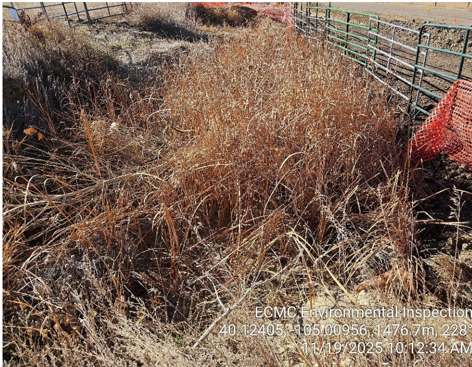
Photo 7 – Weeds in open excavation
