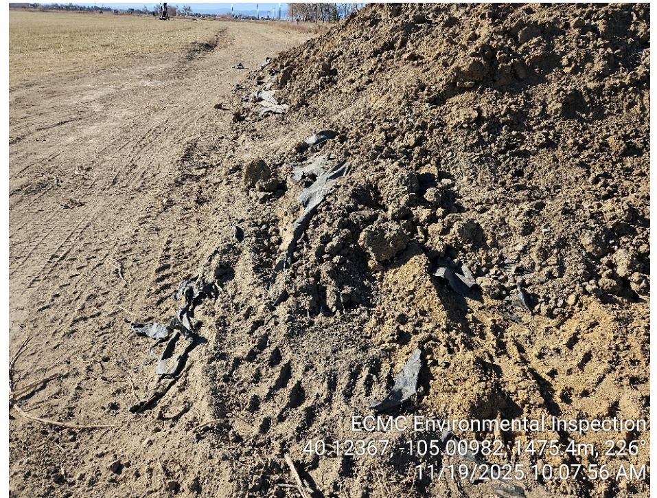
Photo 12 - Soil stockpile. Liner is torn. Stormwater BMPs missing/inadequate.
