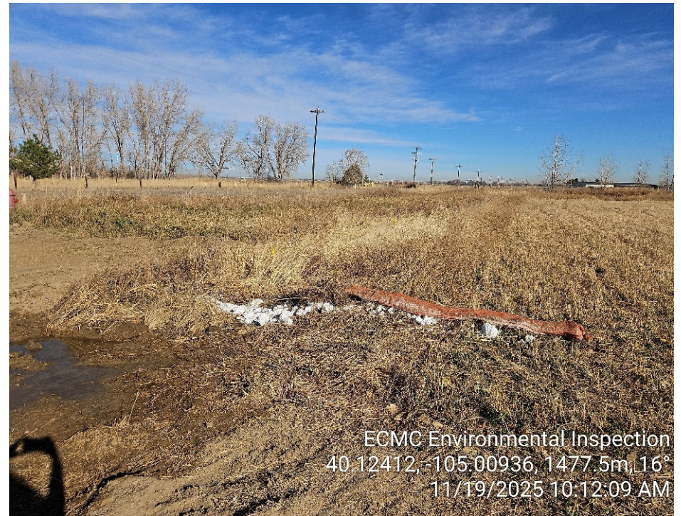
Photo 18 - Stormwater wattle has degraded and become trash.
