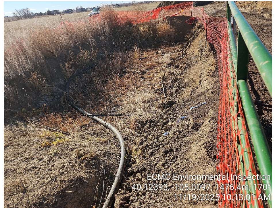
Photo 8 - Open excavation. Weeds in and around open excavation. No groundwater present. Flowline exposed.
