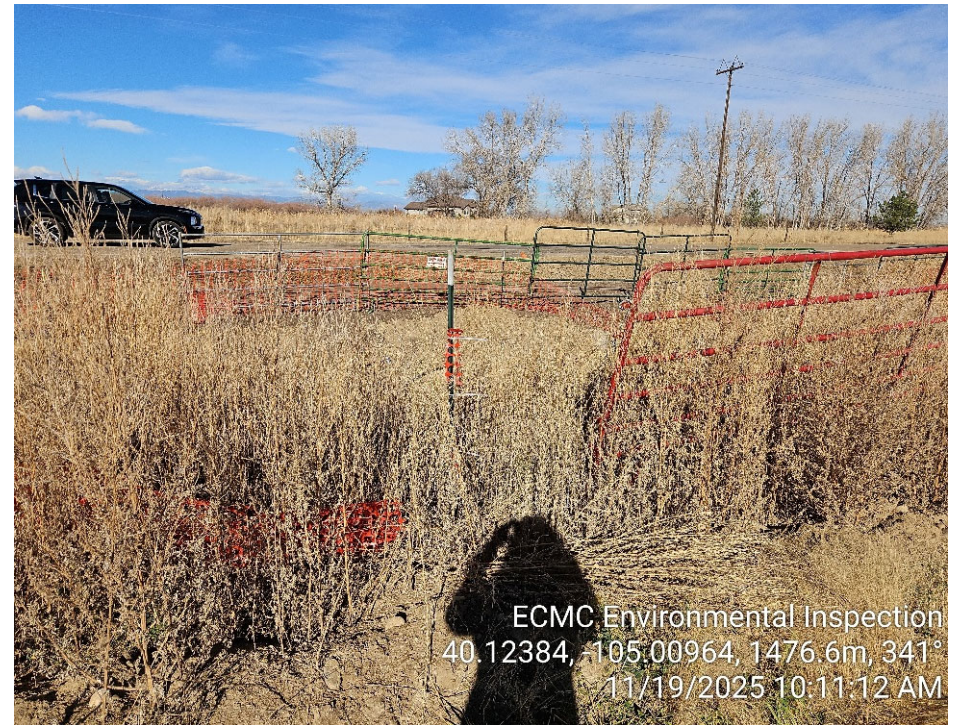
Photo 10 - Fencing down in portions of the excavation.
