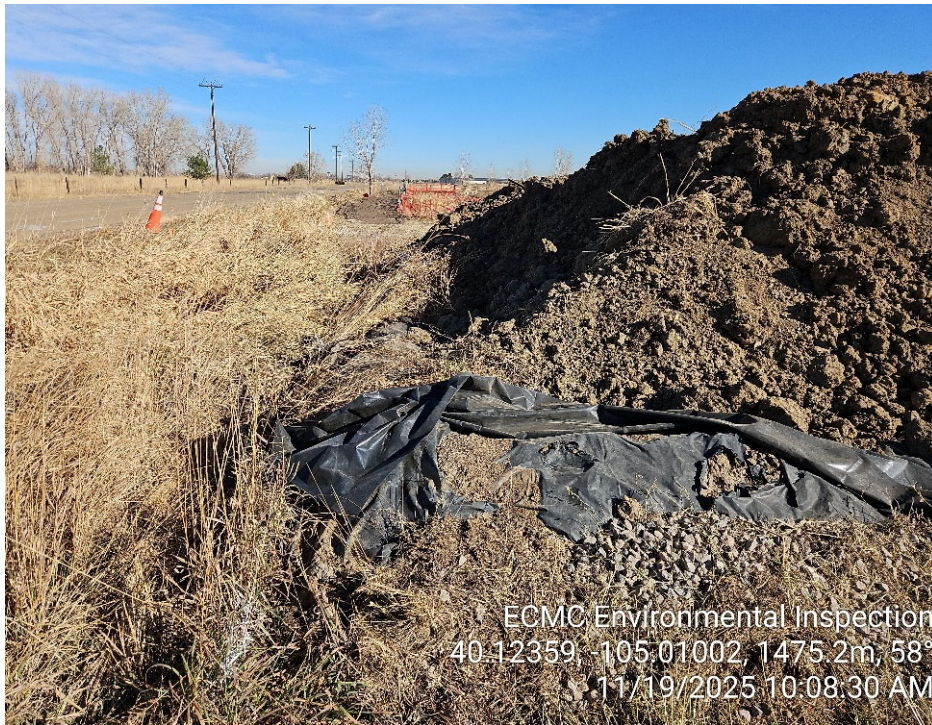
Photo 17 – Soil stockpile. Stormwater BMPs missing/inadequate.
