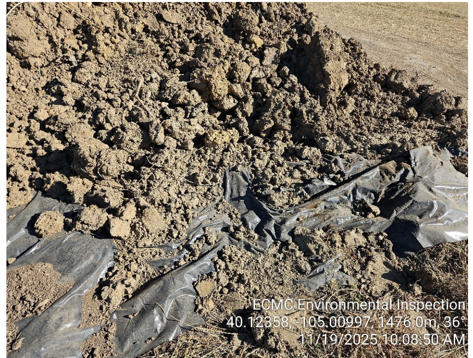
Photo 16 - Soil stockpile. Stormwater BMPs missing/inadequate.
