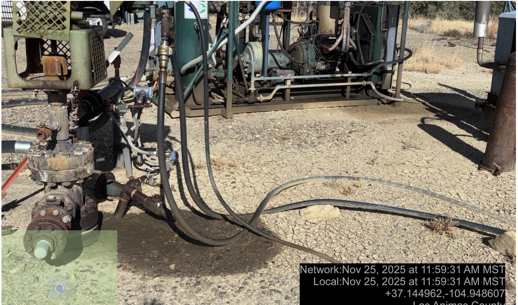
PHOTO 4: Impacted soil identified near wellhead and compressor skid. Conduct maintenance on equipment, cleanup stained material and review self inspection processes. COMPLY WITH RULE 1002, (2).D. this is the 2 nd notice for this corrective action, immediate action is required.
