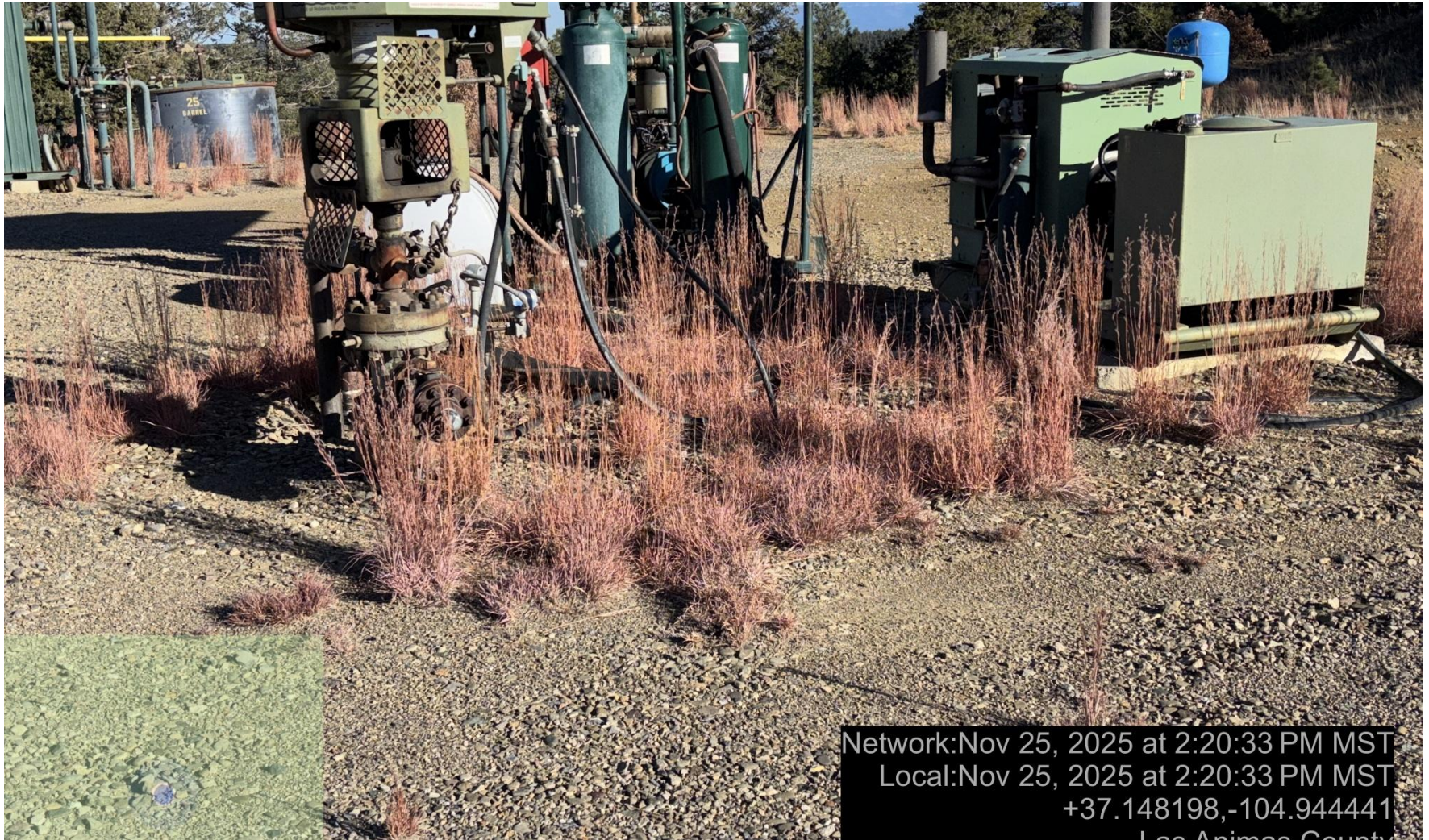
PHOTO 4: WEEDS NOT MAINTAINED NEAR WELLHEAD AND METER HOUSE. MAINTAIN WEEDS PER FULE 606. CA DATE 12-8-2025.
