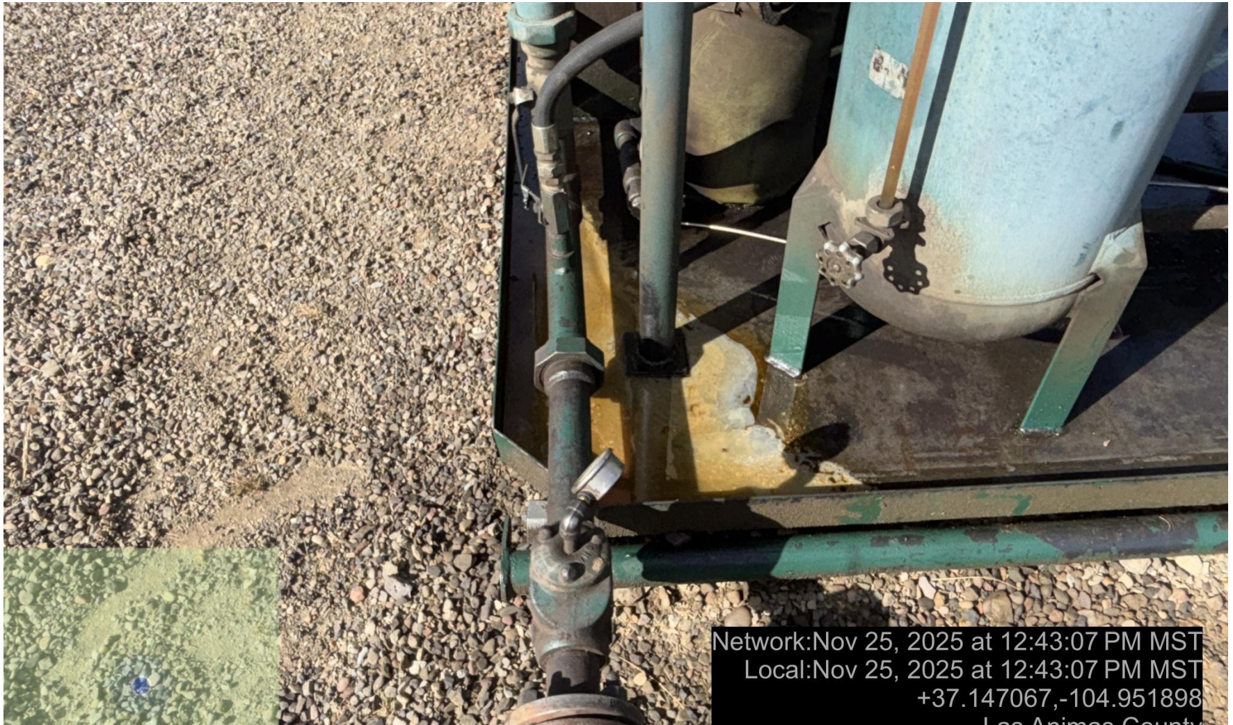
PHOTO 7: OILY WASTE IN COMPRESSOR SKID. DRAIN OILY WASTE REPAIR ALL LEAKS AND REMOVE IMPACTED SOIL PER RULE 1002..(2).D & 1002.f.(2)B, Comply with general provisions of the oil and gas act for wildlife protection AND SB-181. CA DATE 11-26-2025.
