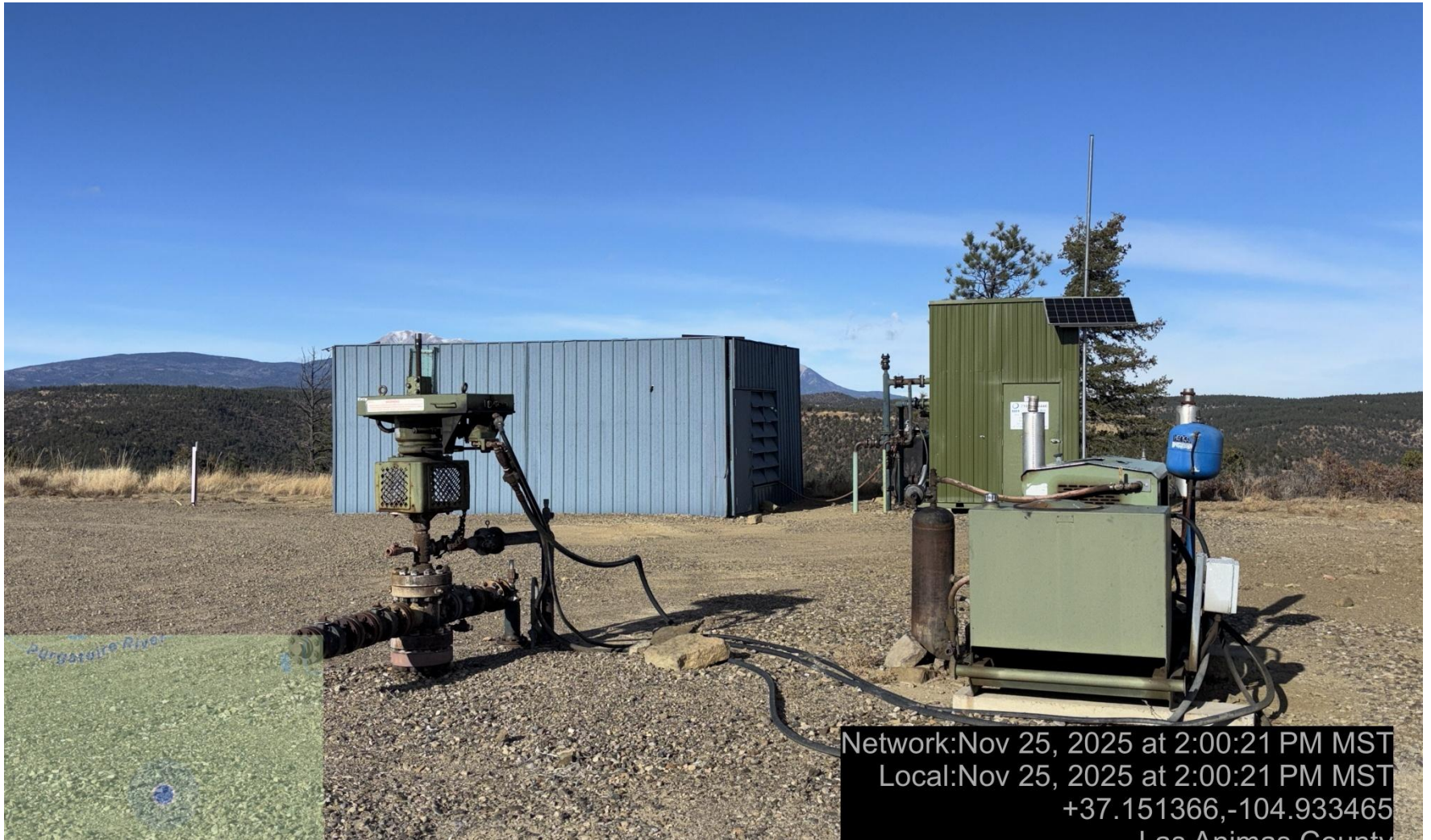
PHOTO 3: WELLHEAD AND EQUIPMENT.
