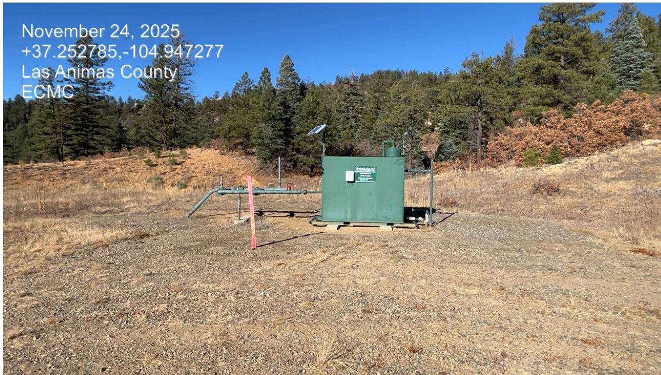
Photo 2. Well sign is posted on meter shed..
