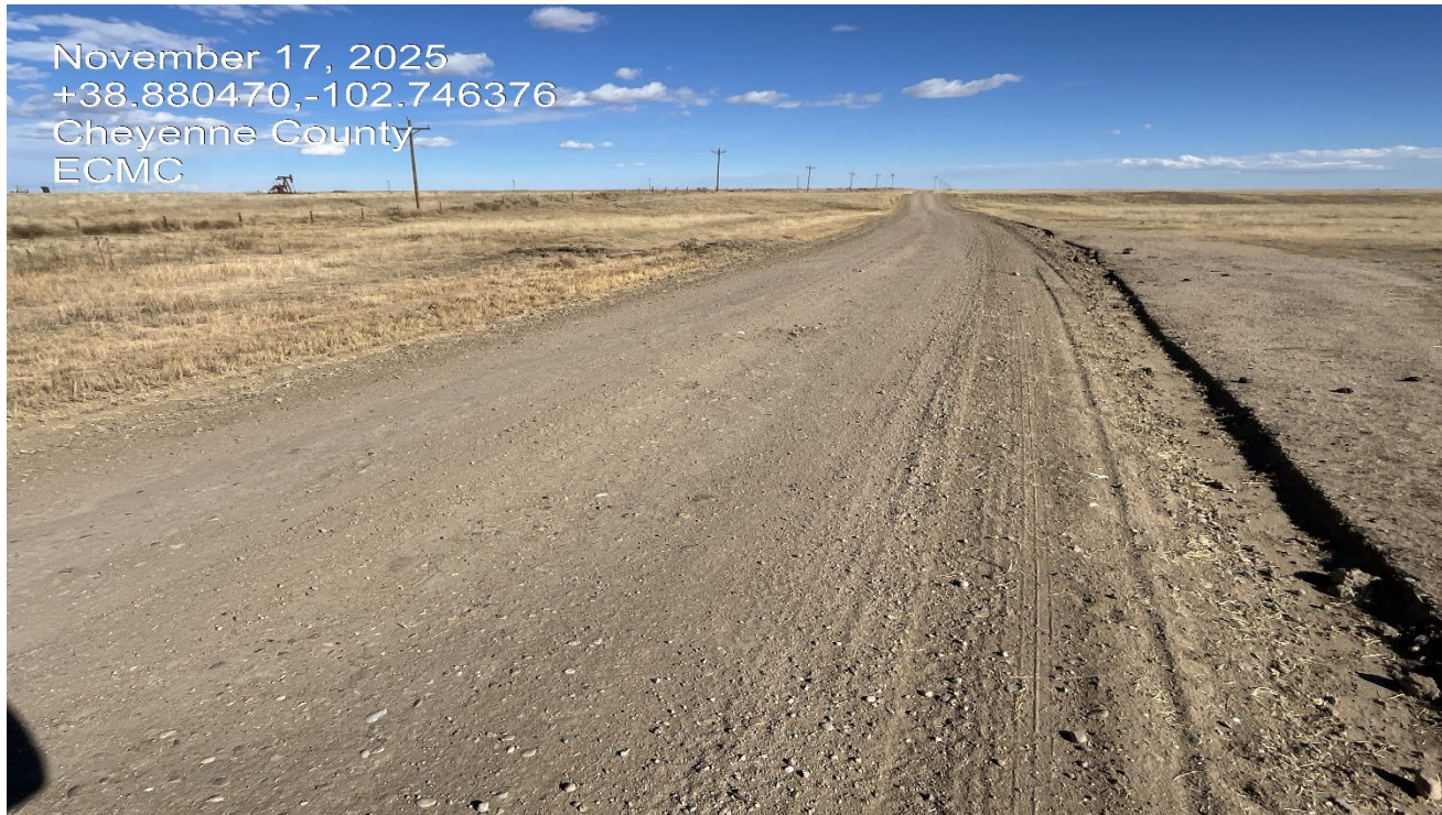
Photo 1. Facing east along the access road. The road has been regraded. The disturbed area where vehicles were driving will need to be decompacted and reclaimed.
