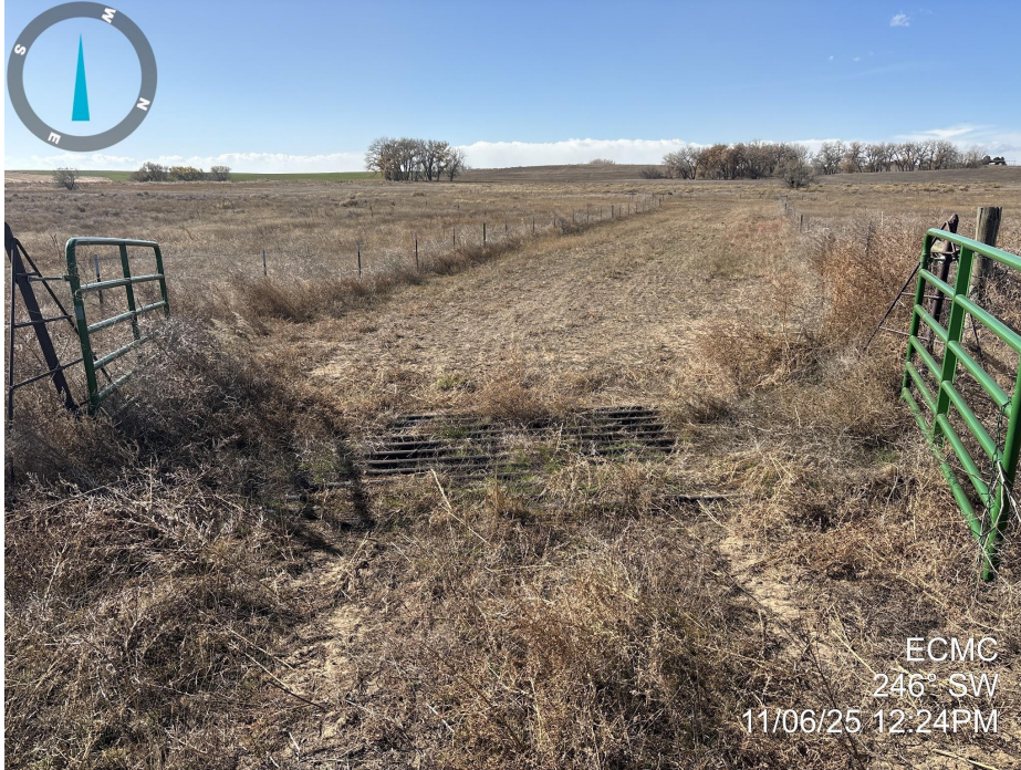
Photo 5. Photo taken of the access road to the location, facing southwest. Photo illustrates that final reclamation activities have taken place, but the cattle guard and fencing remains and vegetation establishment does not meet Rule 1004 standards.
