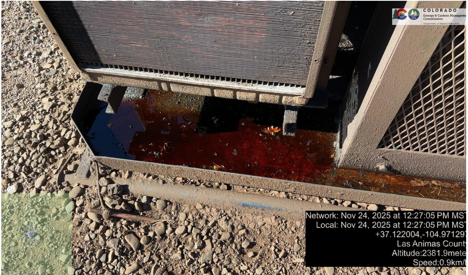
PHOTO 5: OILY WASTE IN COMPRESSOR SKID FROM LEAKING EQUIPMENT. DRAIN OILY WASTE REPAIR ALL LEAKS AND REMOVE IMPACTED SOIL PER RULE 1002..(2).D & 1002.f.(2)B, Comply with general provisions of the oil and gas act for wildlife protection AND SB-181. CA DATE 24 HOURS REMOVE OILY WASTE, FIX LEAKS BY 12-28-2025.
