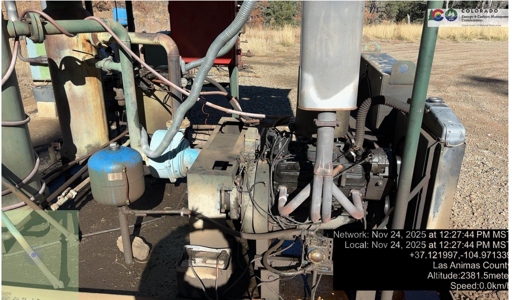
PHOTO 6: OIL SATURATION ALL OVER COMPRESSOR SKID.
