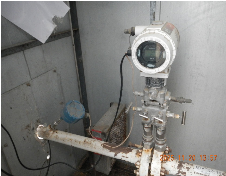
5. Gas Meter inside Meter Shed.
